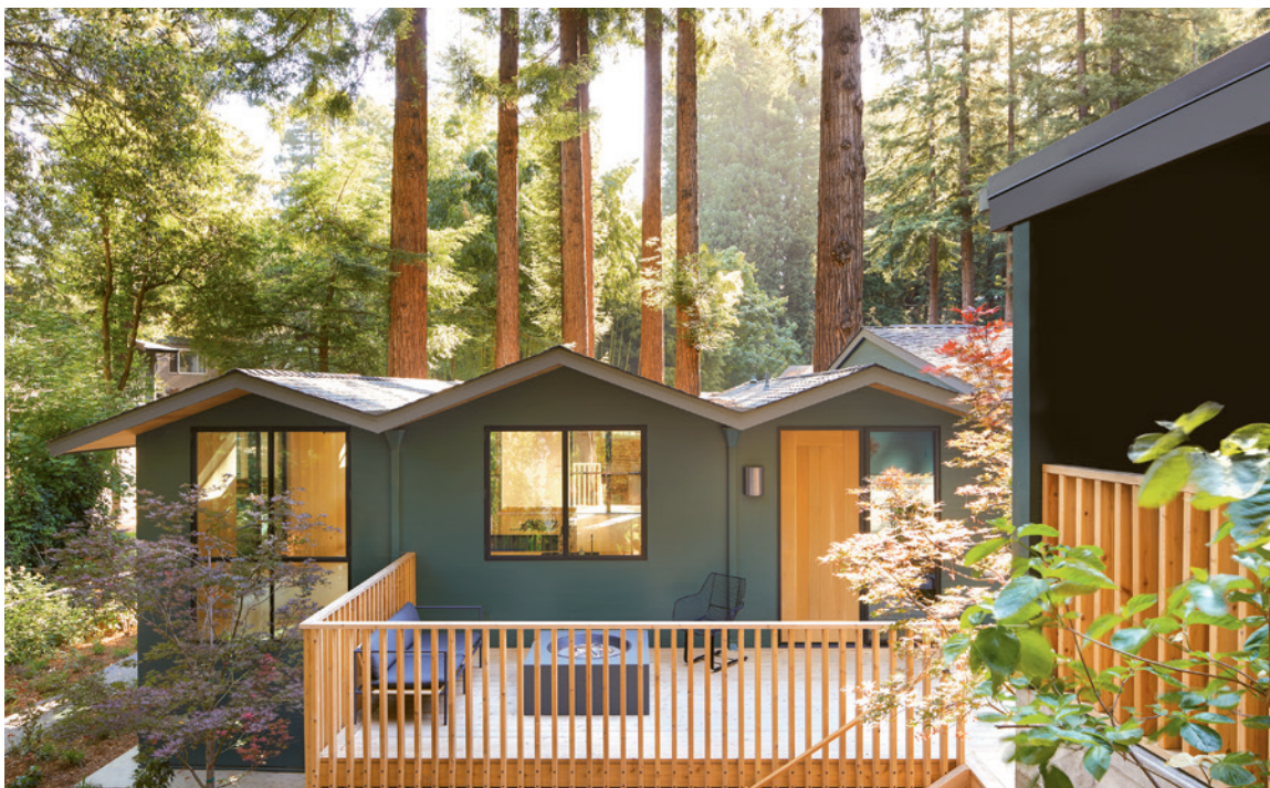
This page: Renovating this former log cabin from the early 20th century was more about removal than addition. The biggest moves: restoring its original third gable and reorienting the front entry.
