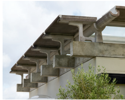
This page and opposite: The skylight's original concrete framing and water channels evoke Japanese detailing. New slotted windows open sight lines between the atrium and the bedroom wing, and between a sitting nook and the Lawrence Halprin-designed pool terrace, now partly restored.
