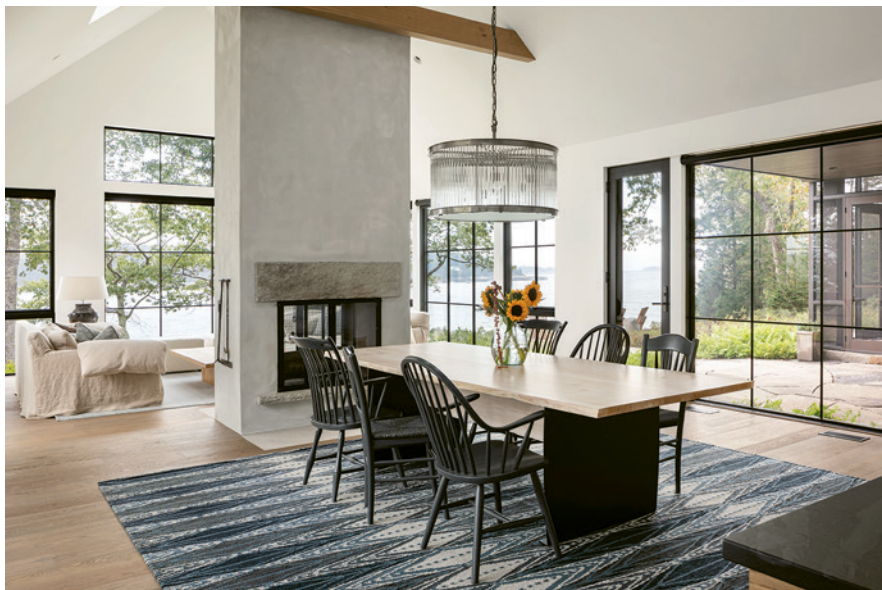
This page: There was no question the original living room/dining room had to come down, as windows and doors were just 2 inches taller than the client. With a raised top plate, new 8-foot windows open the room fully to light and views.
