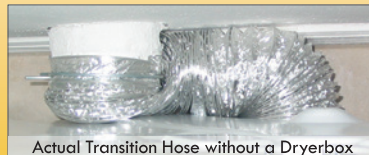
Actual Transition Hose without a Dryerbox
