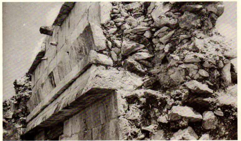
9. Edzná, view of binder molding in veneer facing over concrete rubble core.
