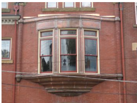
NIKO Contracting Co., Inc. fabricated and installed this custom copper radiused bay window surround.
