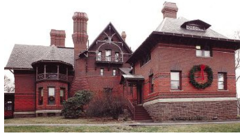
Kronenberger & Sons restored the exterior of the Mark Twain House Museum in Hartford, CT, a job that involved masonry raking and re-pointing.
