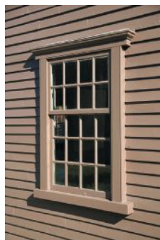
Architectural Components restored the windows for the Jacob Whittemore House at the Minuteman National Historic Park in Lexington, MA.
