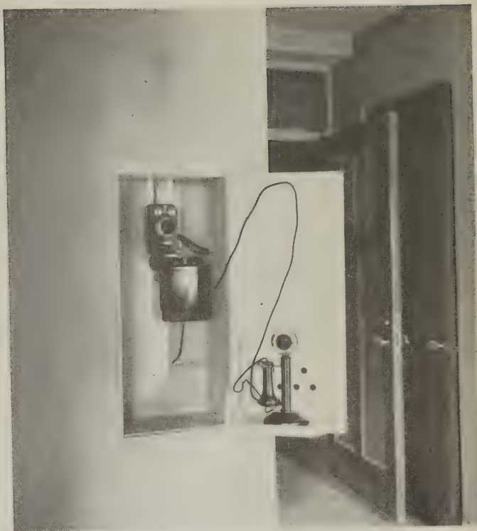
Telephone cabinets are provided in each apartment
