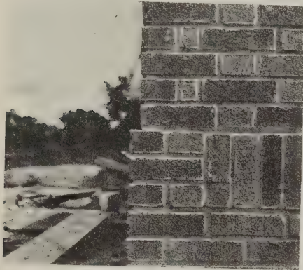
This corner is correctly built and will stand
