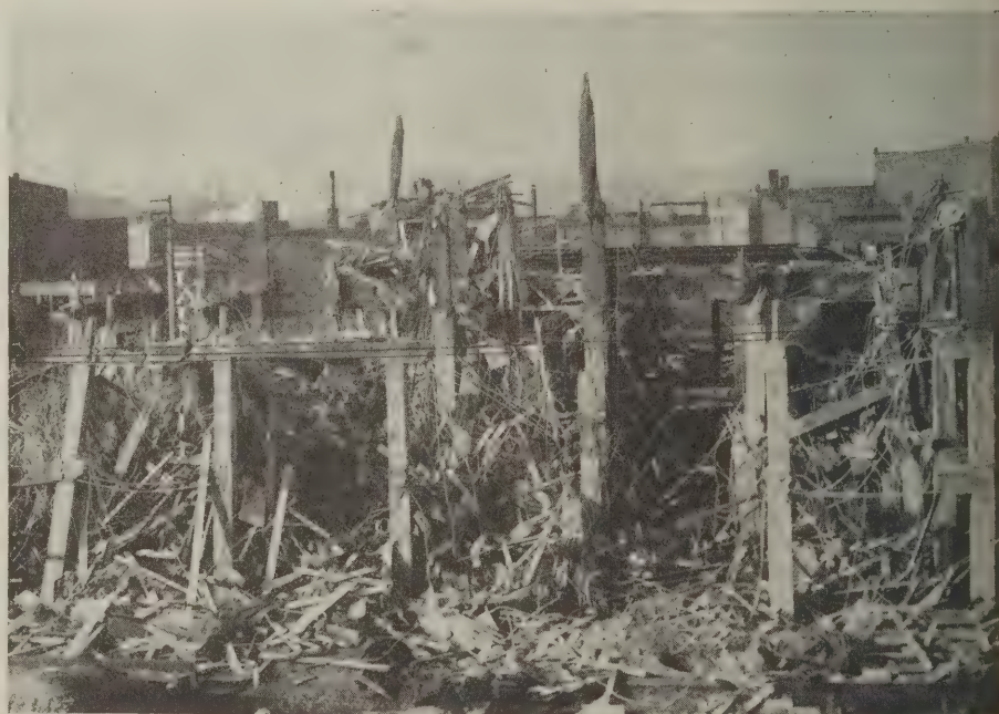
Fig. 2. This illustration shows the structure after the collapse was complete. Only a few of the first and second floor columns remain standing
