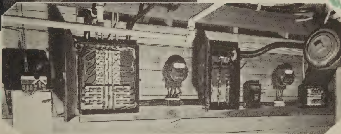
Separate meters, fuse boxes, and safety switches are used—one group for light, the other for power
