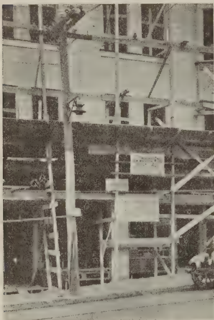
This sidewalk protection is fastened to the scaffolding posts. It is inclined toward the building so that any debris falling upon it will not roll off to the street
