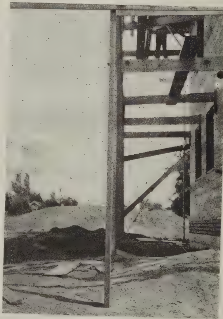
An unsafe scaffold leg. It is liable to slip
