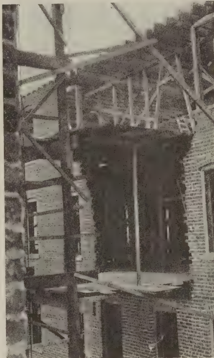
The walls around the delivery platforms were left broken out, to be finished when the elevator was no longer needed
