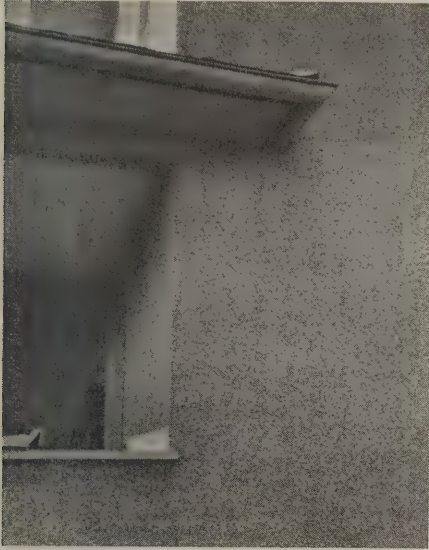
Notice that no cracks are visible under or near the cornice
