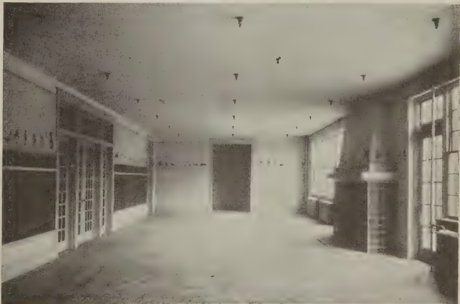
Fig. 6—The tots in this kindergarten are protected by more than a score of automatic firemen who are always on duty
