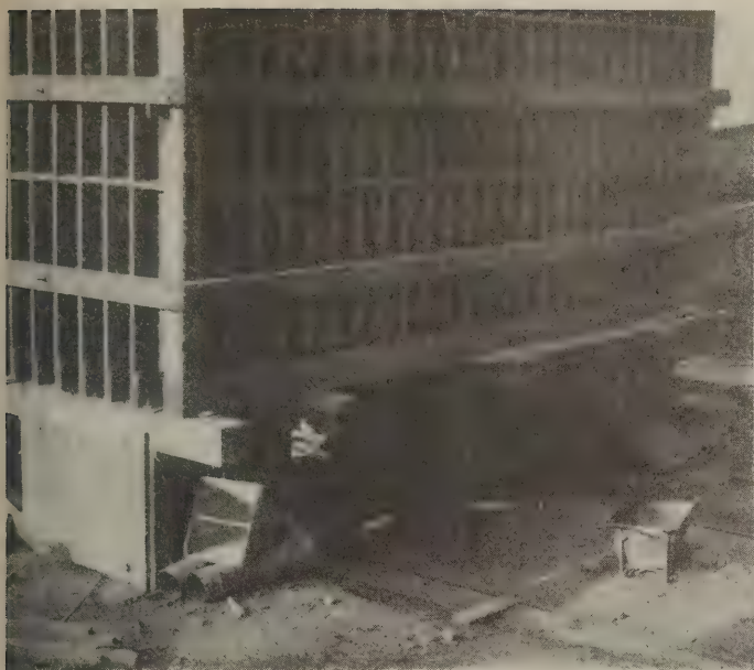
Sidewalk side of aggregate bins showing tracks leading to mixer hopper
