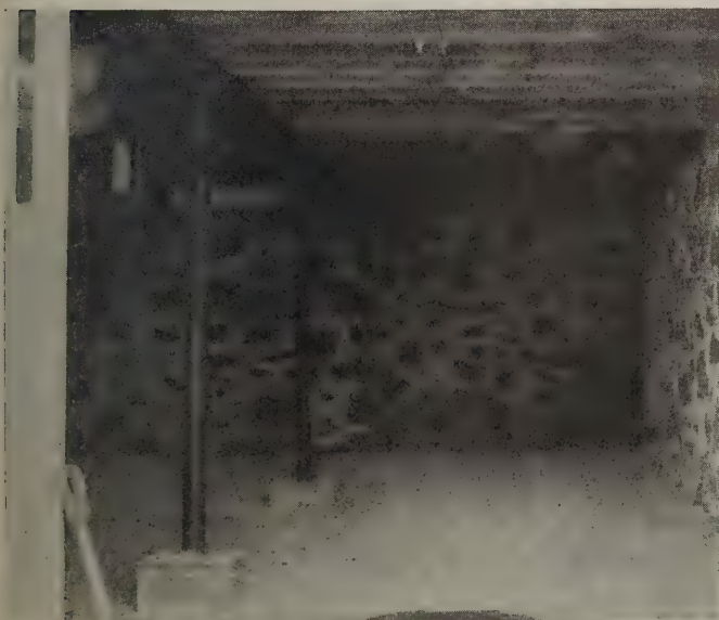
Cellar-garage detail, showing sump under car stand for draining wash water
