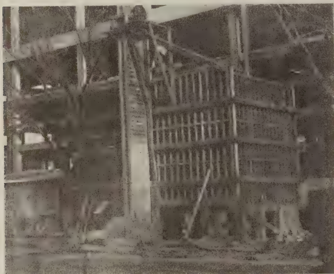
Receiving bin for sand and gravel aggregates
