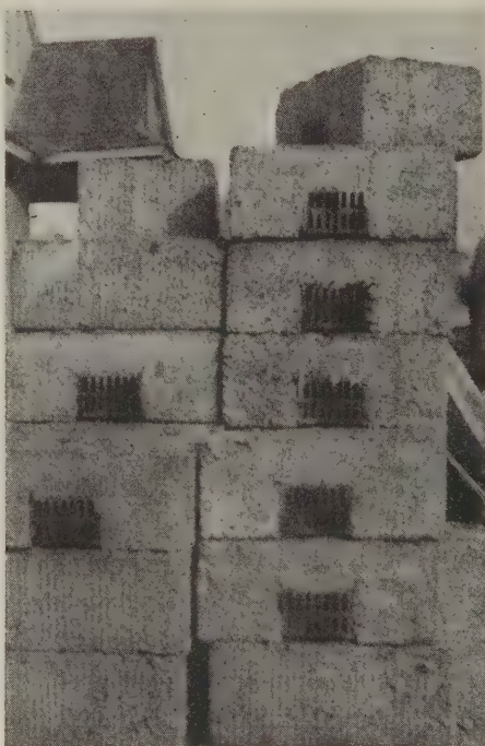
The use of these ventilating blocks proved successful in preventing moisture on the inside walls
