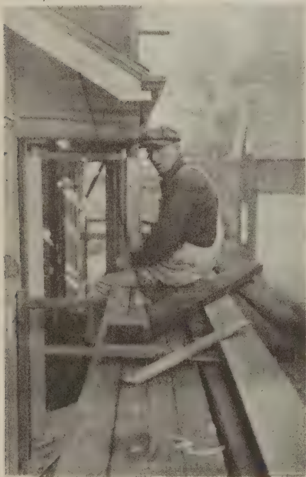
Plate 2—This scaffold is rendered highly dangerous on account of the litter of loose planks, some of which contain bare nails.
