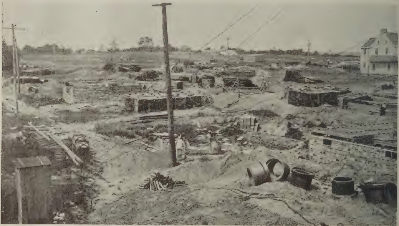
Hollow tile is used extensively for industrial housing developments
