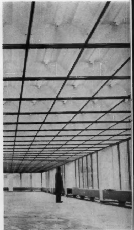
4. Ceiling system, Union Carbide Corp.
