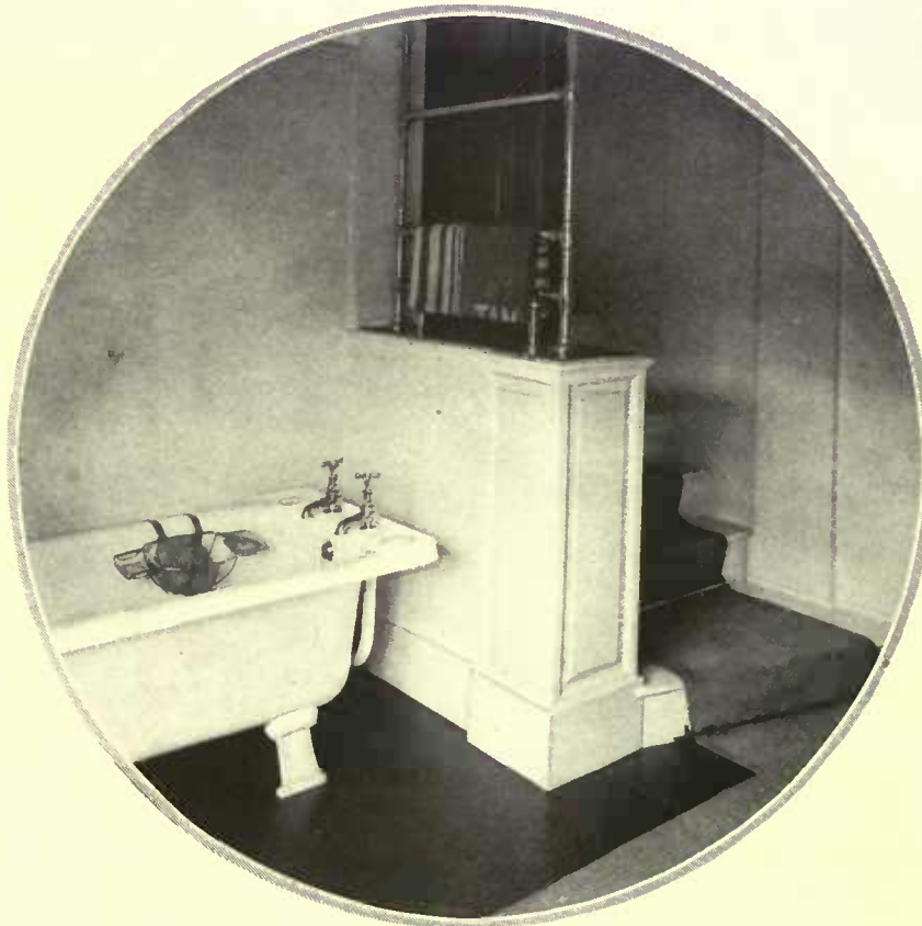
From the English we might well learn the trick of using the steam pipes for a towel drying rack. Here the radiator is concealed in the paneling beside the steps and pipes extend above it. The top of this paneling can have an open grill
