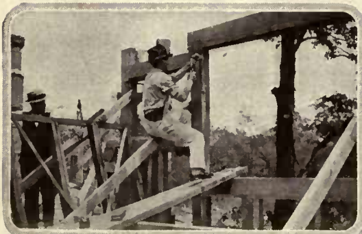
In this stage the first floor timbers are in place and the carpenter is cutting a groove into which to set the window frame
