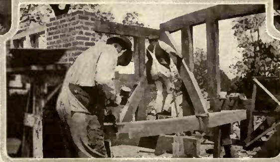
The small photograph above the center shows the joint completed with sheathing and building paper on back of the timber
