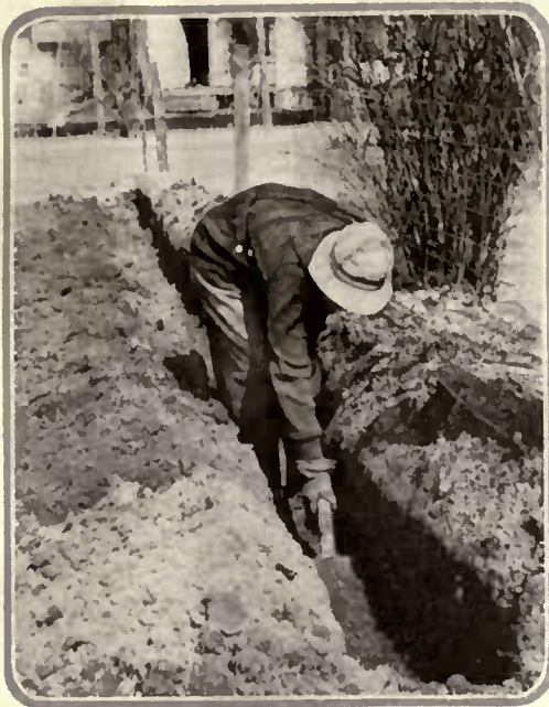
The trench should be dug two spades deep, the top soil being placed on one side and the subsoil on the other
