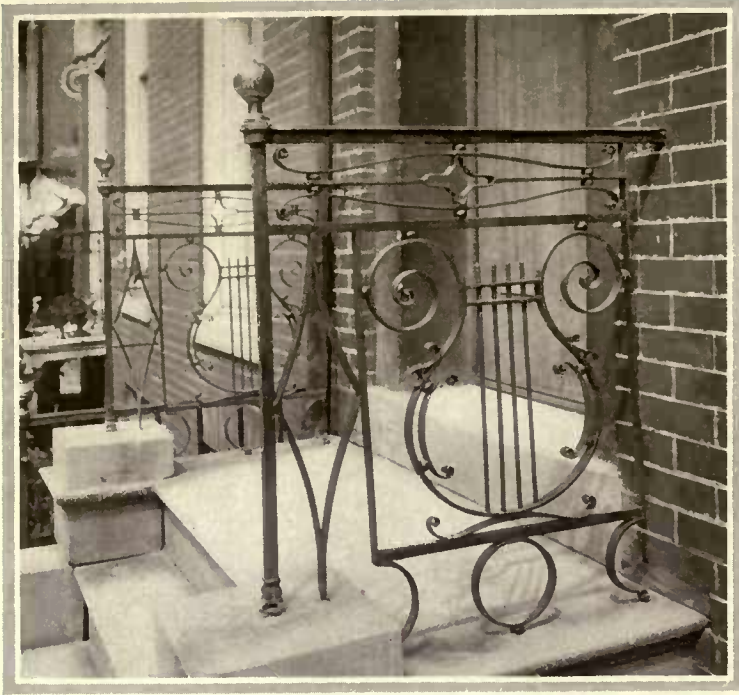
Among the designs prevalent were the lyre motif and the geometrical figure, both of which are combined in this railing to an old Baltimore residence
