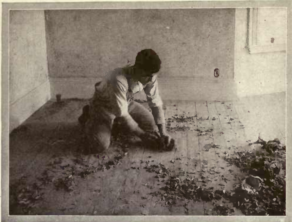
Hard-wood floors require a level sub-floor. They should not be laid until the plastering is thoroughly dry and all the other woodwork in the room finished
