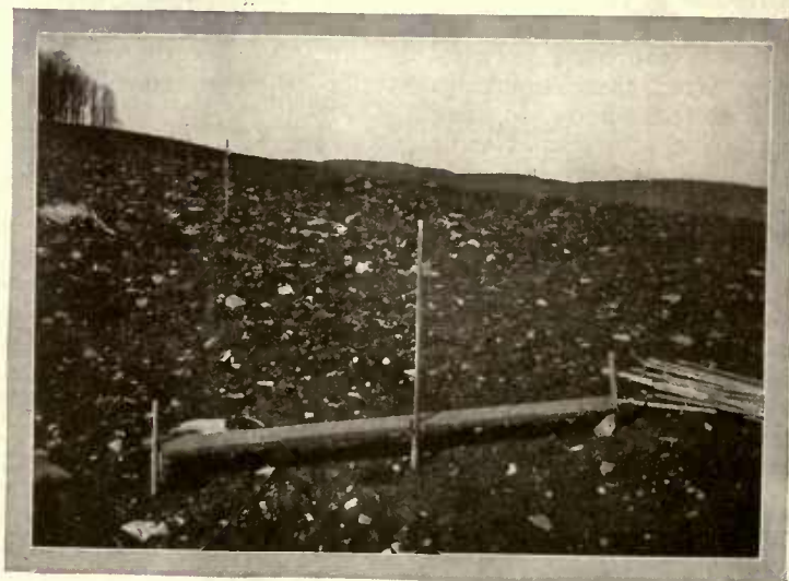
In order to set trees in exact lines, a home-made measuring tool was used. It pivoted on a center pole which swept the possible circumference of the trees
