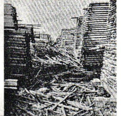
Construction site materials waste and surplus stock.
