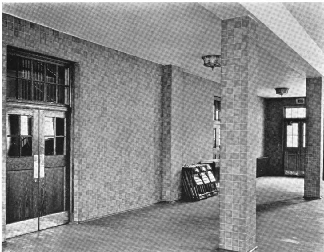
AUDITORIUM OF "M" STREET SCHOOL, WASHINGTON, D. C. Municipal Architect, District of Columbia, Architect Walls and columns faced with 4x4 brown fire flashed ceramic mosaic tile
