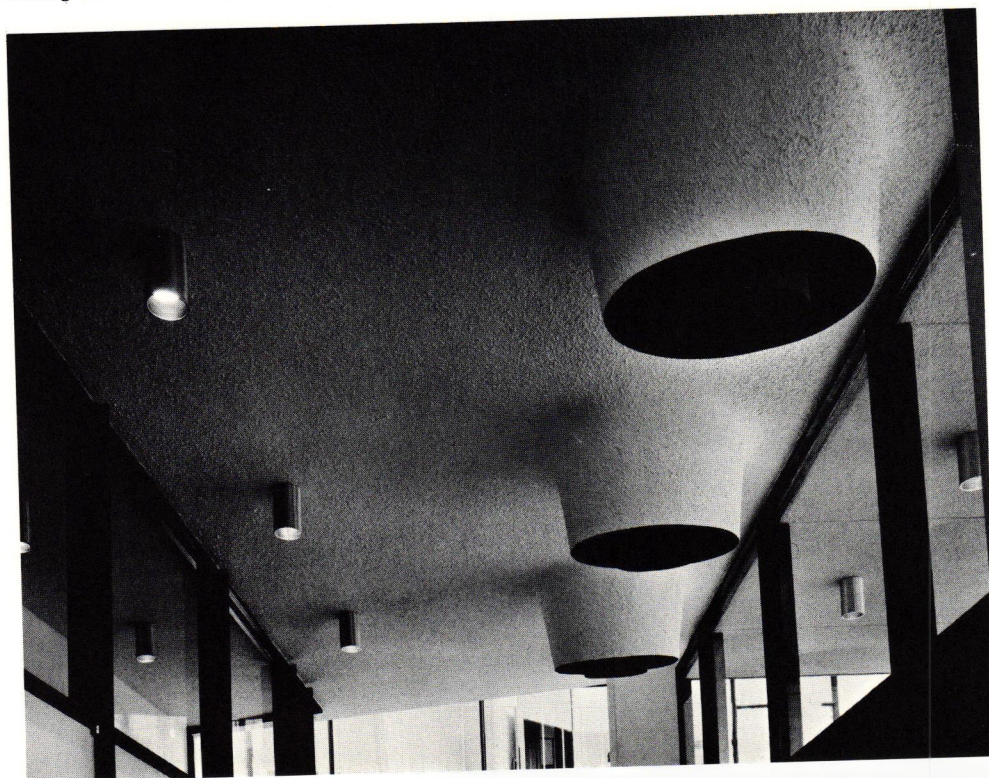
Ceiling air conditioning and heating units above front entrance.
