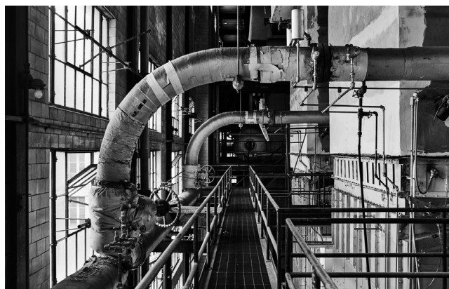
09 Isadore Rosenfield with Starrett & Van Vleck, Archs, Roosevelt Island Power Plant, New York, USA, 1936, catwalk to the boilers. © Charles Giraudet, 2015.
