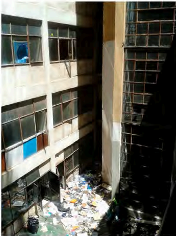
Image 2 – The internal courtyard after the building was high jacked by tenants (Photograph courtesy of Mayat Hart Architects)
