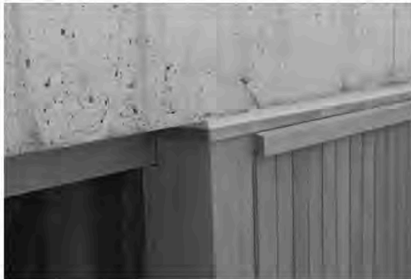
Figure 5. Salk Institute for Biological Studies, La Jolla, California, USA, 2017. View of low-profile metal flashing and sealant inserted at the top of the window head assembly. © Wiss, Janney, Elstner Associates Inc., 2017.
