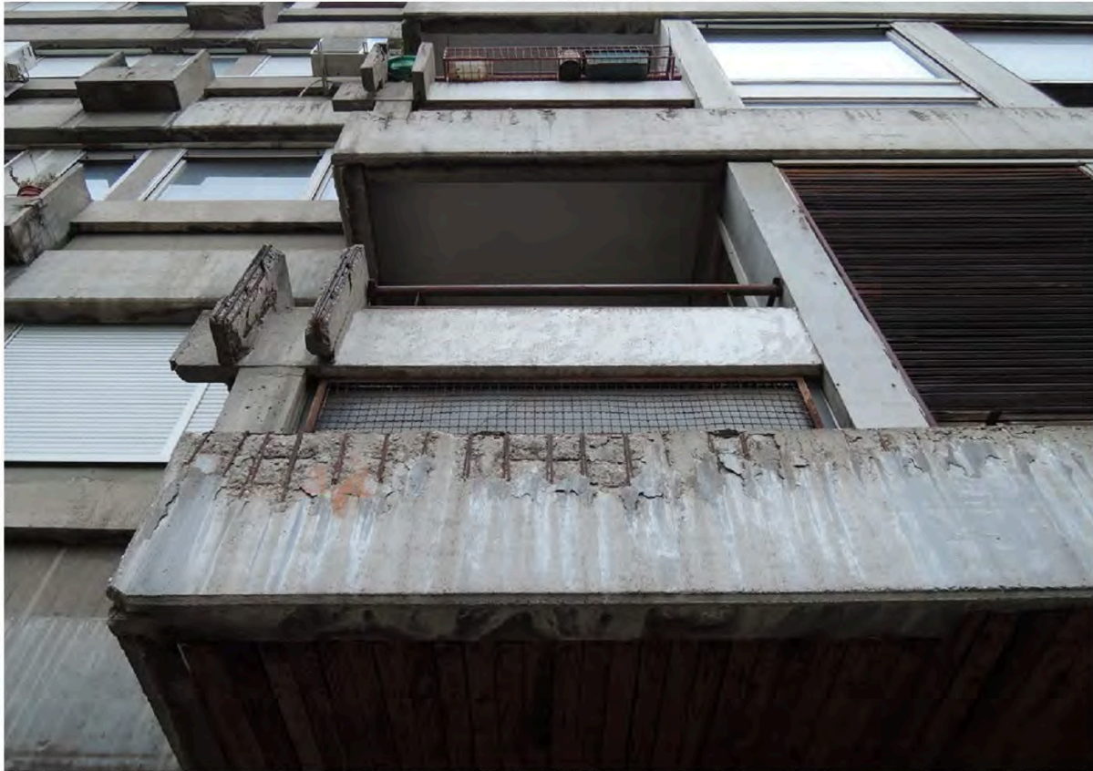
Facade of the meander No. 9 - delamination, corrosion of the reinforcement (photo by Jelica Jovanović, February 2018)
