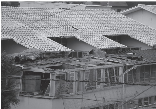
04 Matsumura Masatsune, Hizuchi Elementary School, Yawatahama, Japan, 1958. Roof of the corridor of the East Building was blown away by a typhoon in 2004.
