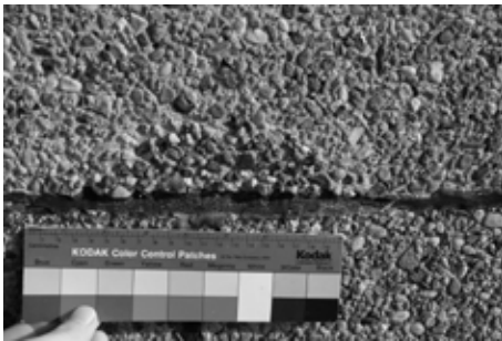
Fig. 5 De Geus & J.B. Ingwersen, Eerste Technische School, Amsterdam (NL), 2013, after restoration, showing detail with a half-moon shaped patch repair above the colour reference grid. Photo: Wessel de Jonge architecten.
