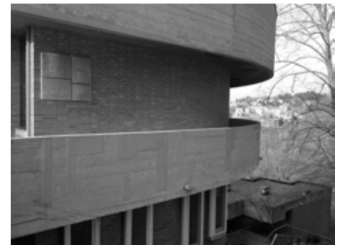
Fig. 3 Giancarlo De Carlo, Collegio del Colle, Urbino, Italy, 2014, the fair face concrete repairs by De Carlo. (Canziani)”
