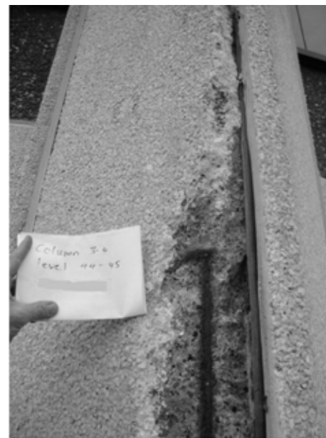
Fig. 3 Australia Square Tower View of the outboard edge of a column panel after removal of a spall of white concrete caused by corrosion of the steel reinforcement in the panel. Source: Preservation Technologies, January 2012
