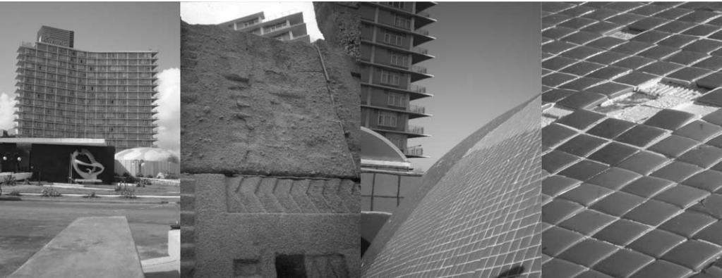
Figure 1. Degradation of Ornamental Mortar Panel and Glass Tile Veneers exposed to Tropical Marine Environment at Havana Riviera Hotel High Rise Building.
