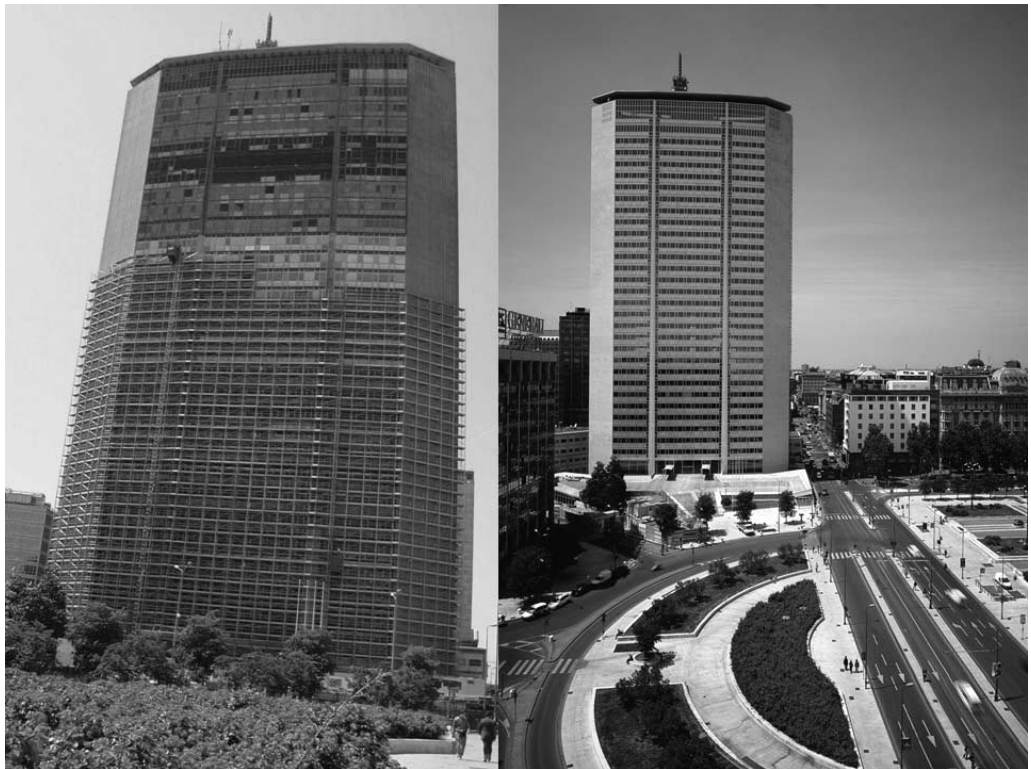
Figure 2. The skyscraper facade damaged by the air crash, 2002 (Archivio Regione Lombardia), and after restoration, 2004. Archivio Corvino + Multari.
