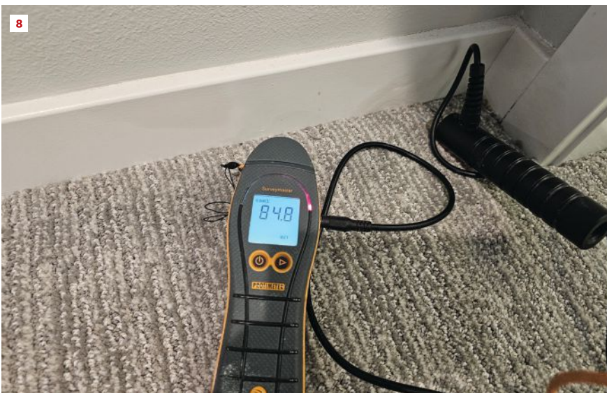
With the probe of the moisture meter buried in the floor sheathing beneath the carpet, the author found levels between 70% and 85% MC.
