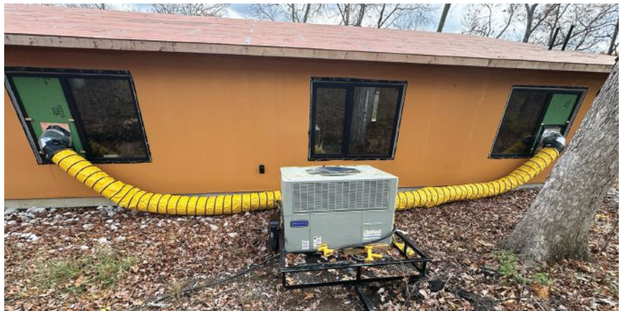
Jake's onsite AC not only improves conditions for the crew but also helps productivity.
