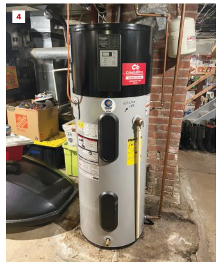
Heat-pump water heaters recover more slowly than gas-fired units. In retrospect, this unit should have been upsized.
