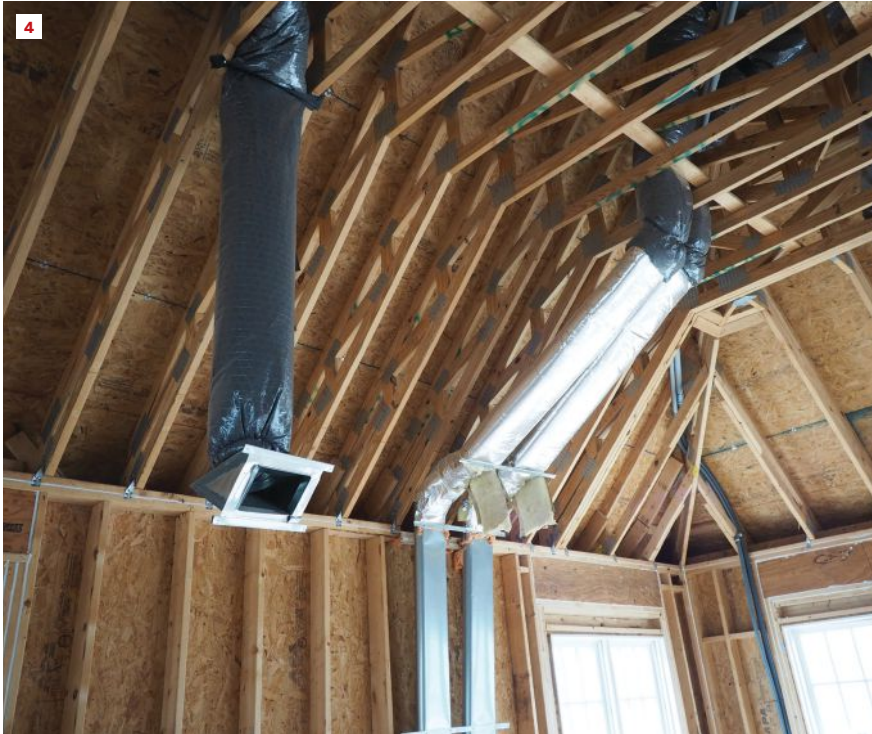
At left in the photo above, a section of flex duct and boot has pre-attached straps for final installation after insulation. At right, two rigid metal ducts are similarly set up with straps that will be used to attach the duct after the cavities have been insulated (4).
