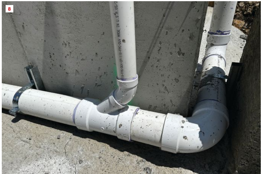
The American Concrete Institute does not directly address plumbing embedment. Playing it safe, the author kept all plumbing and perimeter drainage above the flowable fill (8).
