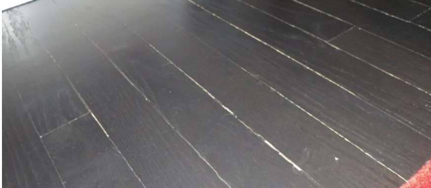
In an especially cold January (2025), shrinkage gaps between oak floorboards were a frequent callback. The dark stain emphasized the gaps.
