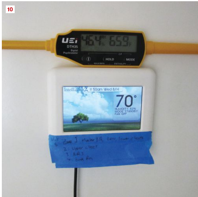
Thermostats can vary from actual temperature and humidity conditions. Here, the thermostat is overstating the temperature by about 4°F and the humidity by about 14%. On most thermostats, the readings can be recalibrated to match a more accurate device.
