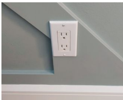
To incorporate this outlet, I added material to fill the space below it.
