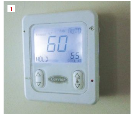
In one case of a miswired damper, the basement AC was running at 60°F in summer, much colder than the set point, and the clients kept lowering the set point because that helped keep the upstairs more comfortable.
