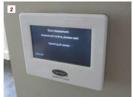
A Carrier zone damper system has a useful diagnostic mode that includes a zone test that opens each zone individually. This allows you to see whether each zone damper was correctly wired to the corresponding connector on the zone control panel.
