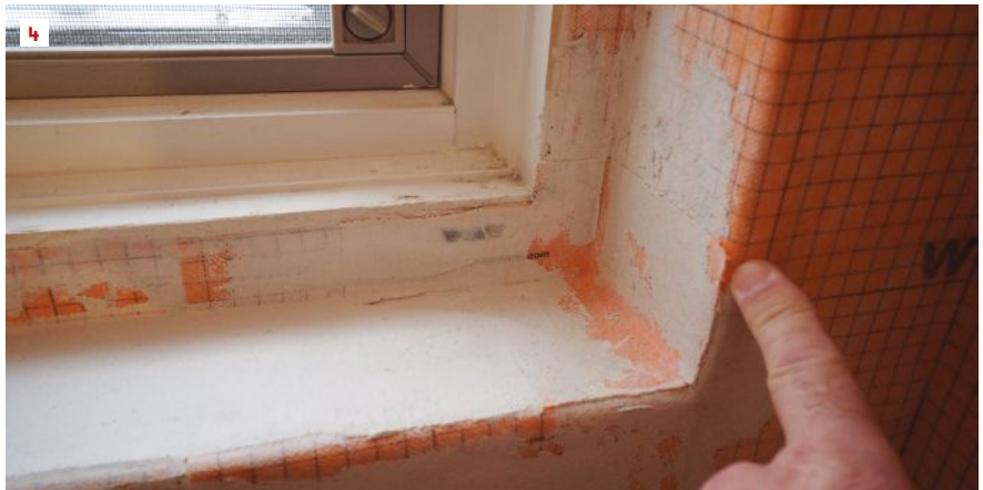
At an existing window in a new shower, the author's company installs Kerdi membrane, lapping it onto the window (2). This application is inherently risky, requiring near-perfect workmanship. The author identifies two instances (3, 4) where the membrane is not sealed and will need extra attention from the crew.
