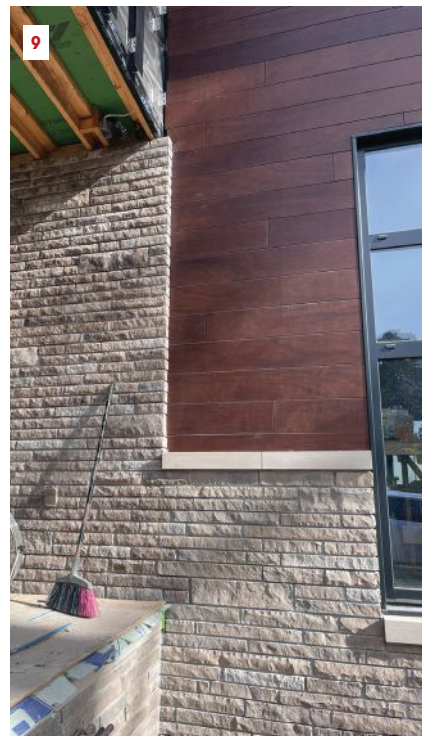
For this vertical transition, the crew had to install the Parklex first, running it long so it would extend behind the stone.
