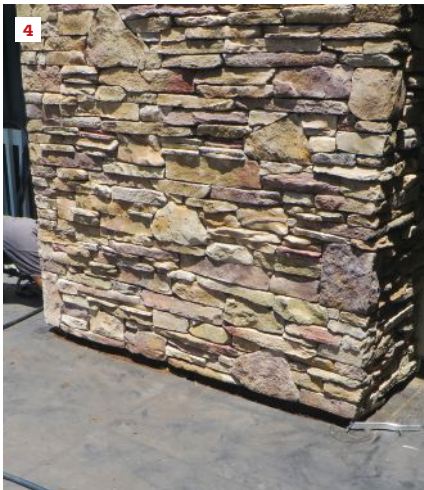
Without a pronounced curb at its base, a chimney can look disconnected from the roof (4). This approach also makes replacing the flashing during a future reroof especially challenging.
