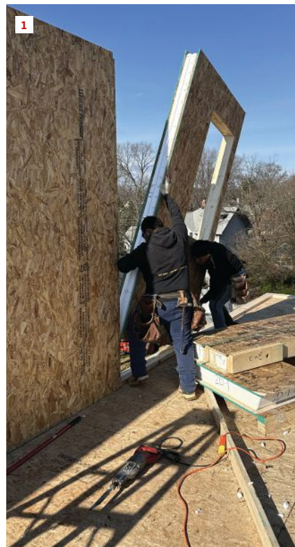
Structure. The Queen of Zero framing crew installs one of 90 structural insulated panels (SIPs) for the home's walls.
