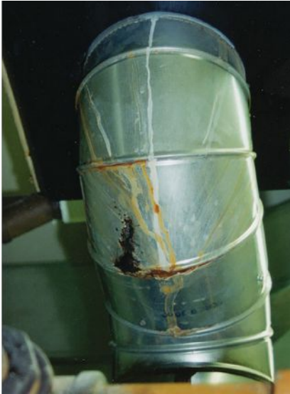
This vent connector had been installed only months before sustained flue-gas condensation caused this corrosion.
