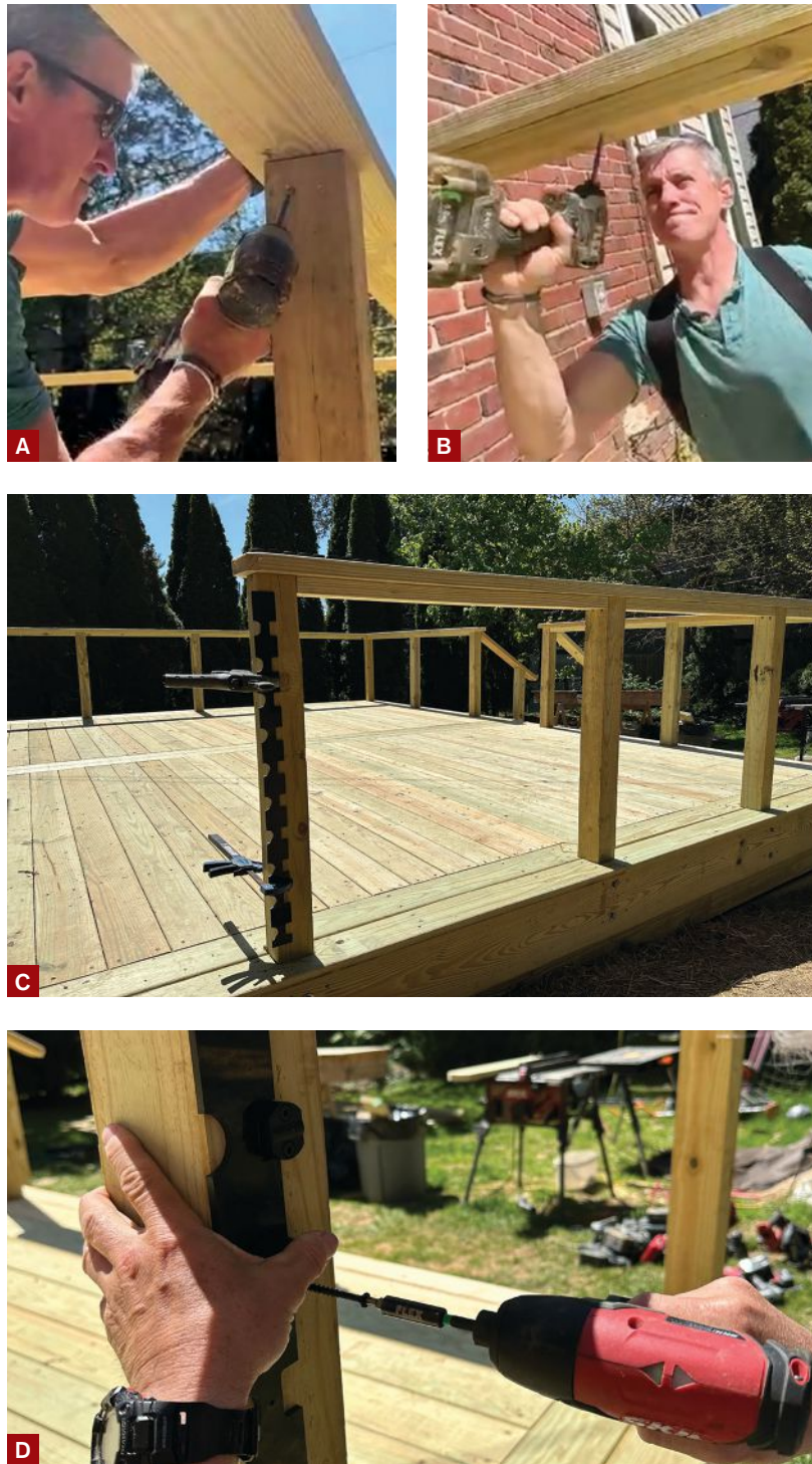
Figure 1. To extend the life of the railing fasteners, the author fastens the top rail to the guard posts from below (A). Between each guard post, he installs a 2x4 subrail (B) to lock the posts firmly in position. This is required to resist the tension the cables transfer to the posts. To streamline the install, he places bar clamps to hold the supplied drilling template to the posts with the bars facing away (C) from where he needs to work with the template (D).
