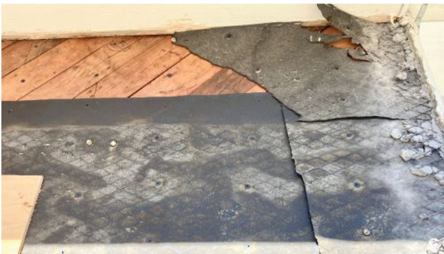
Lumber sheathing. Pictured is a single layer of 30 lb. tar paper torn off a diagonal lumber sheathing wall. Note the demo'd stucco at right. Any air that gets behind the stucco will quickly leak into and out of the wall assembly.
