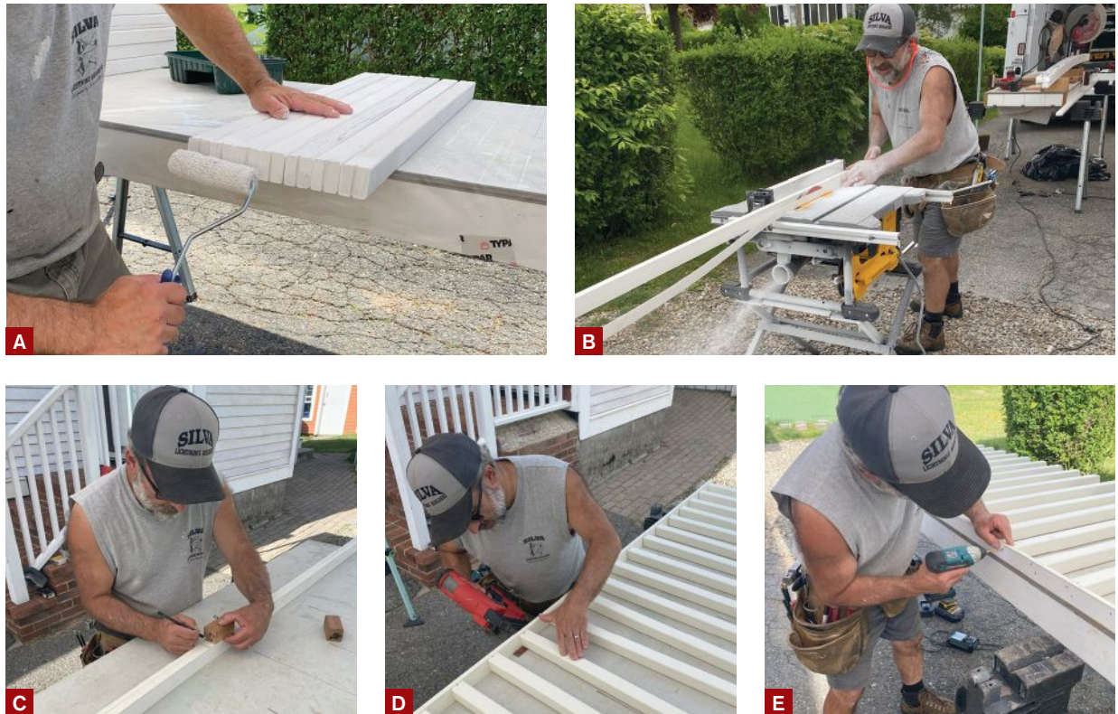
Figure 3. Coating end grain with primer and paint prior to assembly helps prevent the wood balusters from wicking up moisture (A). Here, the author is ripping a 12-degree bevel on one of the PVC nailers (B). After marking the layout from the centers of the upper and lower nailers (C), the author first tacked the balusters to the nailers with 18-gauge nails (D), then strengthened the connection with pairs of 1 1/2-inch trim screws (E).
