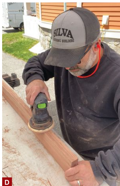
Figure 1. The author ripped a pair of kerfs in the undersides of the 2x4 red balau mahogany rails (A), routed notches in their sides, and then beveled the tops to shed water (C). Prior to finishing, he then sanded them with 100-grit paper (D).
