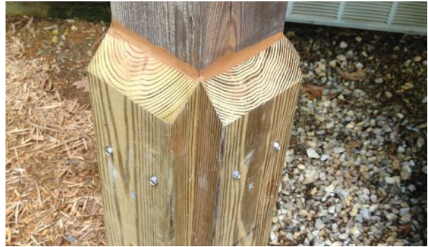
This UC4A-treated 6x6 southern pine post has been repaired using UC4B-treated 2x6 cleats and 1/4-inch-by-3-inch structural fasteners. Note that the cleats (as well as the concrete, not shown) have been sloped to shed water.
