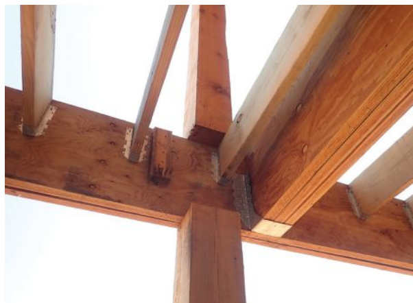
Figure 1. Discontinuous posts don't provide adequate resistance to uplift and lateral forces on a multilevel deck.
