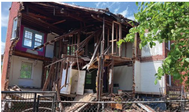
Complete collapse. These photos posted by the D.C. Fire and EMS Department show the tragic consequences of undermining the foundation when digging down a basement.
