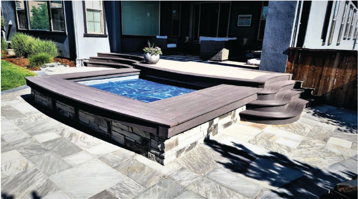
Access to the spa was improved by extending the porch with new TimberTech decking installed over sleepers fastened to the concrete and adding wider curved steps on either side of the spa.
