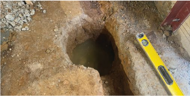
Vertical steel was added prevent the old brick and new concrete walls from hinging (top). The steel precluded the addition of a robust drainage matrix to the walls. Above, the perimeter is prepped for interior perimeter drains.
