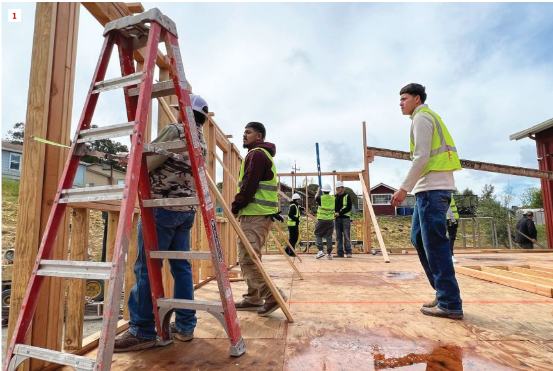
Rancho Cielo students begin framing one of four modules that will comprise Nexus 01, the prize-winning model home that was designed to have a zero-carbon footprint and operate off the grid using solar roofing and storage batteries.
