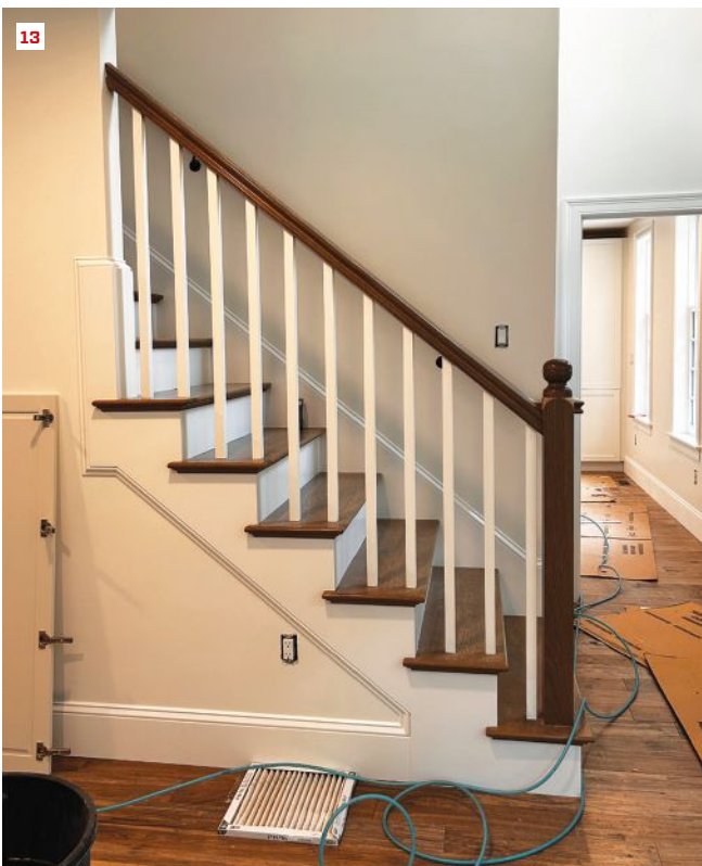
The finished stair with oak bull-nosed treads, newel post, scotia molding (under the tread nosings), handrails, and painted poplar risers, skirtboards, and balusters (13).
