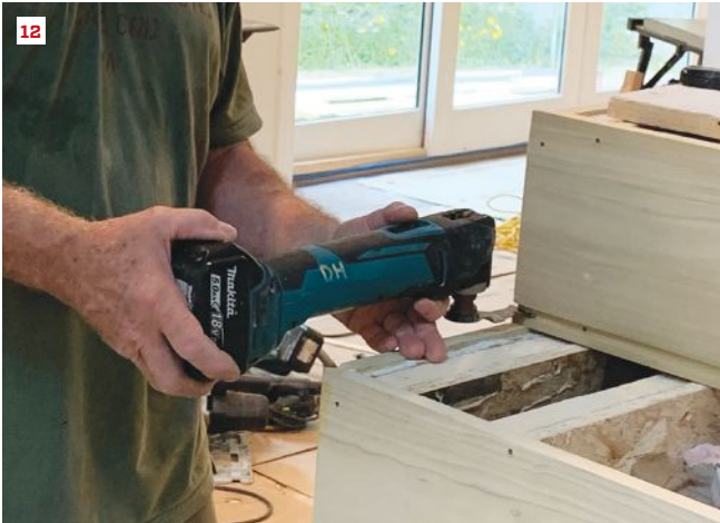
Where the lower six treads have an open skirtboard, the author used a multi-tool to complete the groove in the riser to receive the tongued tread. A portion of the open skirtboard miter is cut away (12).
