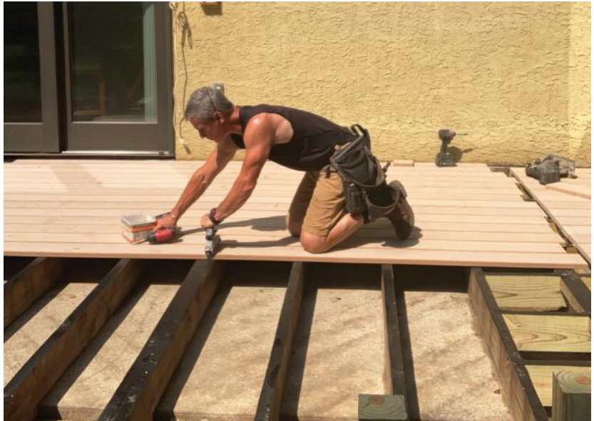
Figure 3. After covering the tops of the joists with self-adhering flashing tape, the author installs the new decking. On this project, he used Modern Mill's Acre decking, a composite material made from upcycled rice hulls and PVC that can be cut like wood and can be stained or painted.
