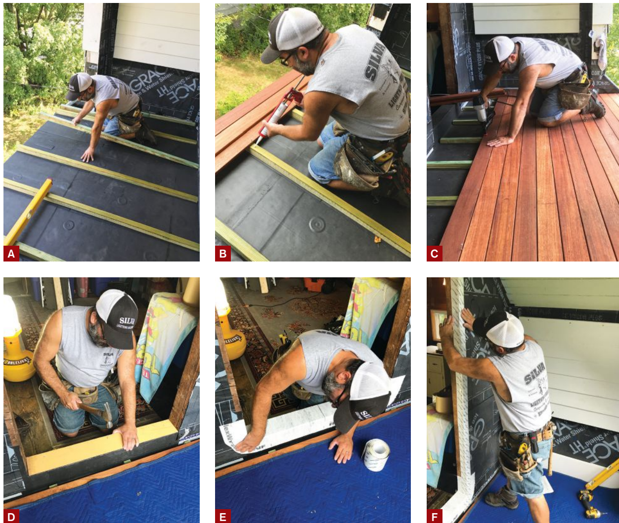
Figure 3. The author laid pressure-treated sleepers with a reverse taper over the membrane (A), then fastened 1x4 red meranti decking to the sleepers with marine-grade adhesive (B) and stainless steel nails (C). At the entryway to the attic, a short length of beveled siding tacked to the door sill over the membrane creates pitch for drainage (D). The author then waterproofed the sill with flexible flashing tape, which wraps up the jambs (E), then used regular peel-and-stick flashing tape to seal the sides of the opening to the WRB covering the wall (F).
