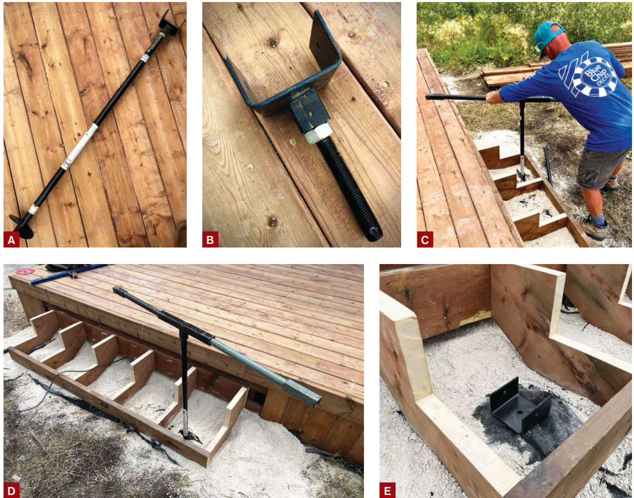
Figure 1. The 50-inch Pylex screw piles (A) with an adjustable saddle (B) that the author uses to support his deck stairs are designed to be installed by hand (C). The manufacturer offers a T-shaped fitting that fits over the shaft of the screw pile; longer lengths of steel rod can be added to the fitting for more leverage (D). Once the pile is embedded in the ground, the adjustable saddle is added to the assembly (E).
