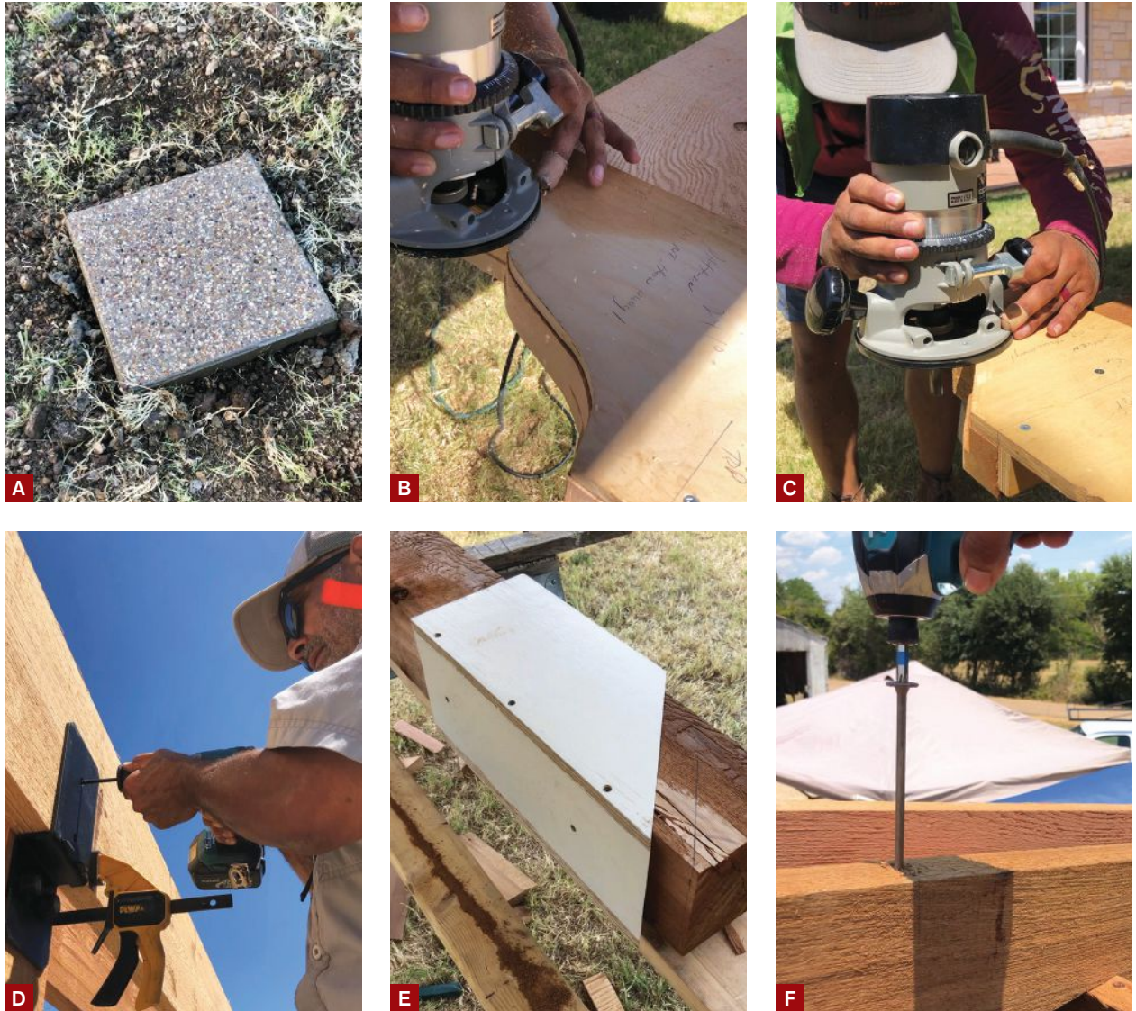
Figure 1. The pergola's support posts bear on the concrete patio and on 16-by-16-inch piers (A). The author uses one jig to shape the ends of the double 2x12 beams (B) and another one to shape the 2x6 rafters (C). Decorative hardware is used to hang the 2x12 beams from the pergola's 6x6 support posts (D). A simple guide made out of scrap material allows the author to make the clean and accurate 45-degree-angle cuts needed for the diagonal braces that reinforce the post-to-beam connection (E). Long structural screws fasten the 2x6 rafters to the beams (F).
