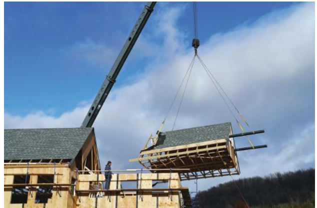
Prefabrication doesn't always need a factory. Lee McGinley found it safer and more efficient to build this roof assembly on the ground and crane it into place.
