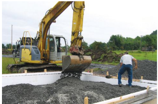
A range of new technologies in residential construction have sped up construction while improving energy efficiency. ICF foundation forms are an example.
