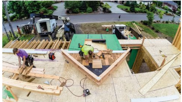
Building faster and safer: Tim Uhler installs the siding, vent, and eaves on rake walls before lifting them in place.
