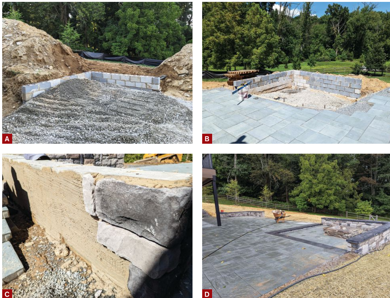
Figure 3. The sitting walls at the corners of the cast-stone-paver patio are supported by full below-frostline footings (A), which prevent heaves and cracks and stabilize the edges of the patio (B). The block walls are finished with manufactured stone veneer (C), and capped with manufactured pavers that match the edging around the sunken fire pit (D).
