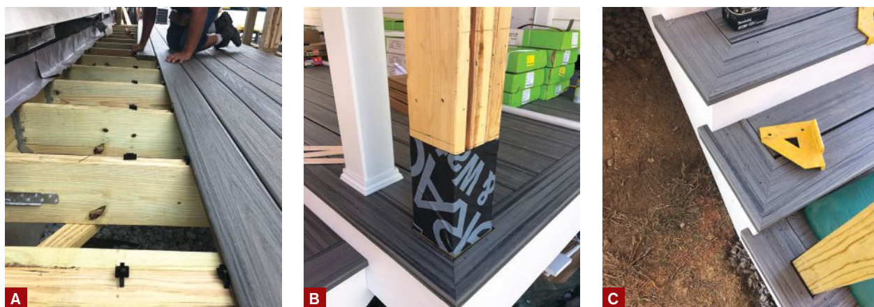
Figure 3. Hidden fasteners were used to install the Trex porch decking (A), while color-matched trim-head screws were used to fasten the picture-framed perimeter edge boards (B) and stair treads (C) to the framing.
