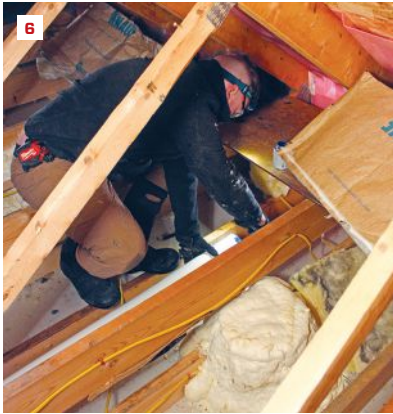
A crew member replaces a length of 4-inch flex duct run from a bath fan with 4-inch rigid PVC piping. The PVC duct sloped 1/4 inch per foot toward the soffit vent. In the foreground, a recessed light is air-sealed with a site-built OSB cover foamed in place (6).
