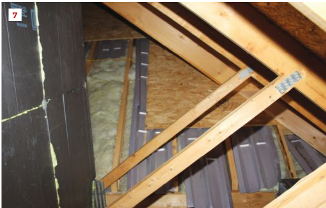
Note the existing ineffective thermal control where the garage wing intersects with the main roof, with large areas of exposed fiberglass and loosely placed Propavents (7).
