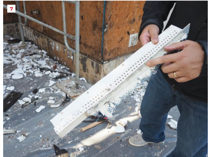
Heavy caulking blocked the weep holes in this plastic track installed at the bottom of the drained EIFS on the wood walls (7). The trapped water caused water staining all along the bottom of the wall, visible in the background.
