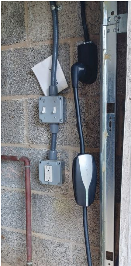
A NEMA 14-50 receptacle wired with a 6-gauge cable running back to a 50-amp breaker in the service panel will work for most mobile connectors.
