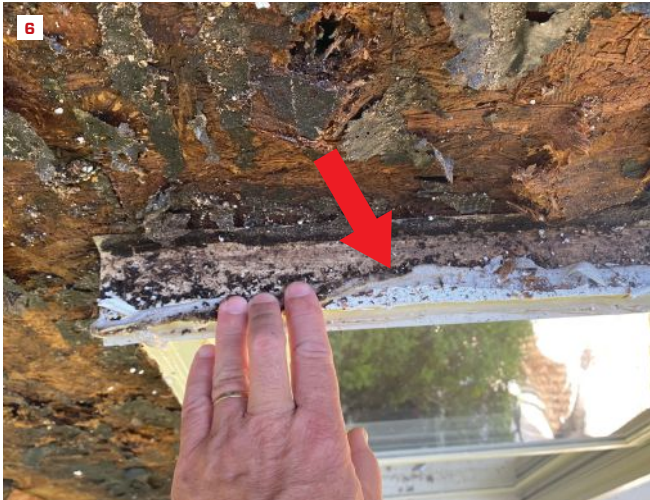
The heavy bead of sealant on top of this window head flashing blocked the drain path from the vertical channels above the window (arrow) (6).
