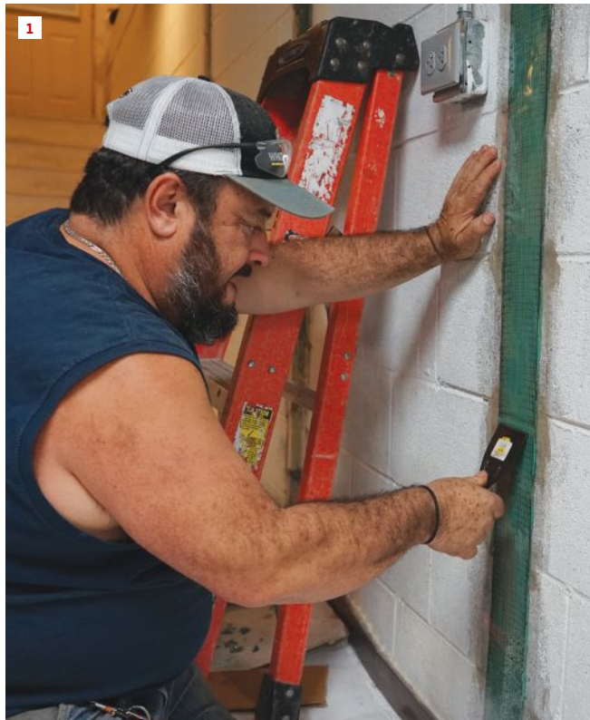
Toby Bonilla of Great Lakes Builders smooths out the two-part epoxy used to reinforce a block foundation wall.
