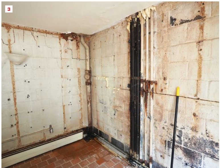
With termite-damaged framing and moldy drywall removed, cracked and leaky block retaining walls were revealed in the interior. Rusted-out electrical conduit and HVAC line sets were also sources of leaking (3).
