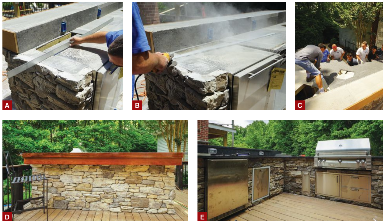
Figure 4. Workers checked the top of the cabinet surface with straightedges (A) and used a grinder to remove high spots (B) to make sure it was flat prior to installing the granite countertop (C). Ipe trim on the bar overhang (D) offers a warm contrast to the stone veneer cladding (E).
