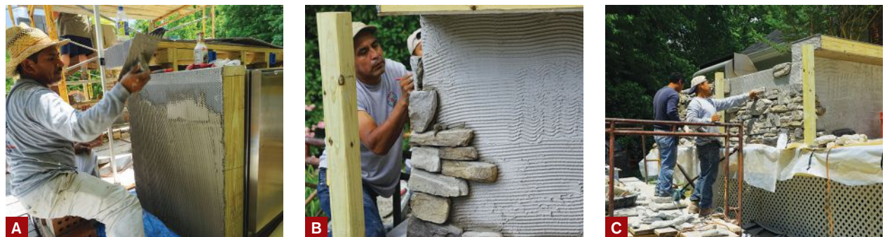
Figure 3. Masons troweled on a mortar scratch coat over galvanized diamond lath fastened to the cement board (A), then allowed the mortar to cure overnight. When applying the manufactured stone veneer, they started at the corners (B) and worked in sections (C), back-buttering each stone and pressing it into the scratch coat.
