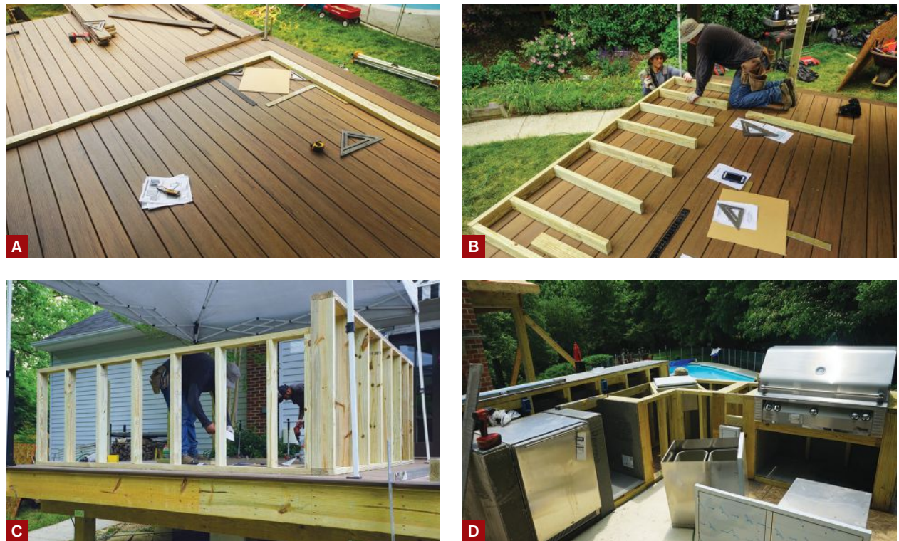
Figure 2. Using cardboard templates sized to fit the appliances (A), workers framed the kitchen's perimeter walls on the deck (B) with pressure-treated 2x4s and 2x6s, then screwed them together and through the decking into blocking installed between the joists (C). The cabinet walls are clad with cement board over a vapor retarder (D).
