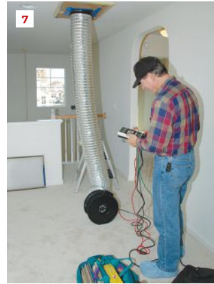
Smooth-wall ducts and all connections sealed with mastic will ensure efficient delivery of supply air (6). And after sealing, every duct installation should be tested for total duct leakage or duct leakage to the outside (7).
