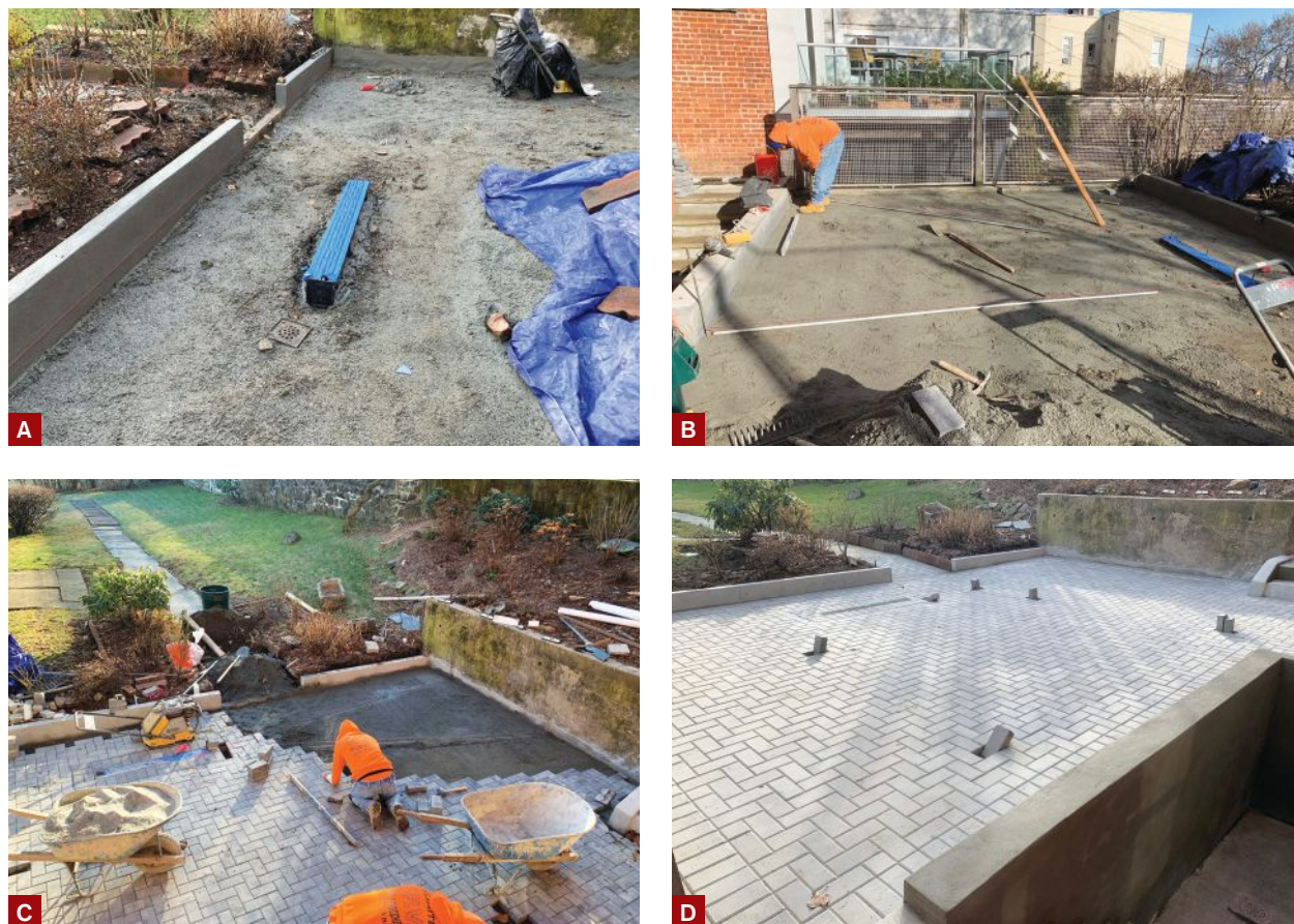
Figure 2. A new linear drain was installed to improve drainage (A), along with a properly sloped QP (quarry process) setting bed for the new concrete patio (B). These measures were needed to capture water draining from the narrow backyard, which is at a higher elevation (C). Upturned pavers mark the locations of the new deck footings (D).
