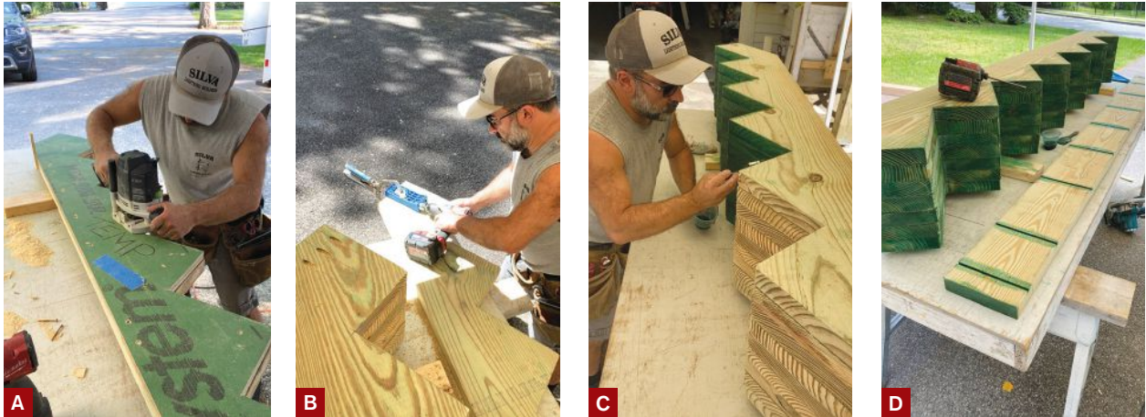
Figure 3. Using a template cut from a double layer of 7/16-inch Zip sheathing, the author pattern-routed the stringers (A). He used a Kreg jig to make pocket holes for mounting screws (B), then screwed the cut stringers together to prevent warping. To prevent rot, he applied preservative to the cuts and notches on the stringers (C) and the landing plate (D).
