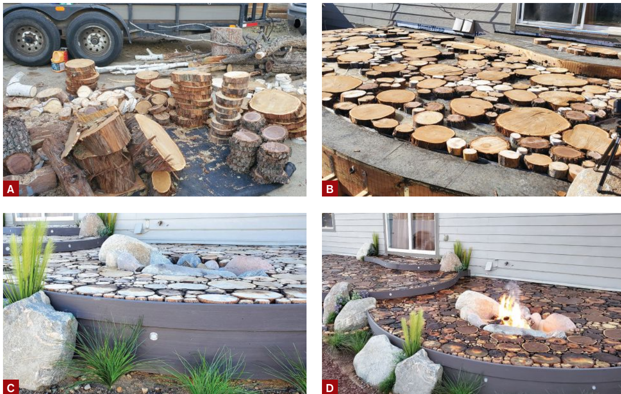
Figure 3. The author cut thousands of log rounds from a variety of sizes and species of wood for the decking (A). During installation, he used screws to hold the larger rounds in place and filled between them with smaller pieces, which were held in place with epoxy (B). After planing and sanding the surface smooth, the author continued to coat the assembly with more coats of epoxy, and wrapped the edge of the deck with composite fascia material (C, D).
