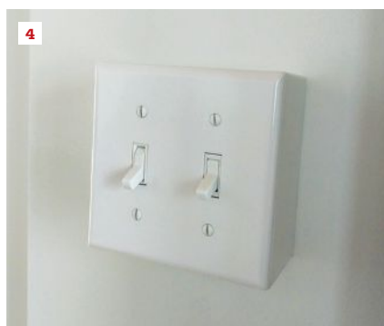
Surface-mount outlets, cable, and Ethernet can be integrated with baseboard (3). The surface-mount wall switch (4) is an example of a fixture on an exterior wall that avoids wall penetrations.
