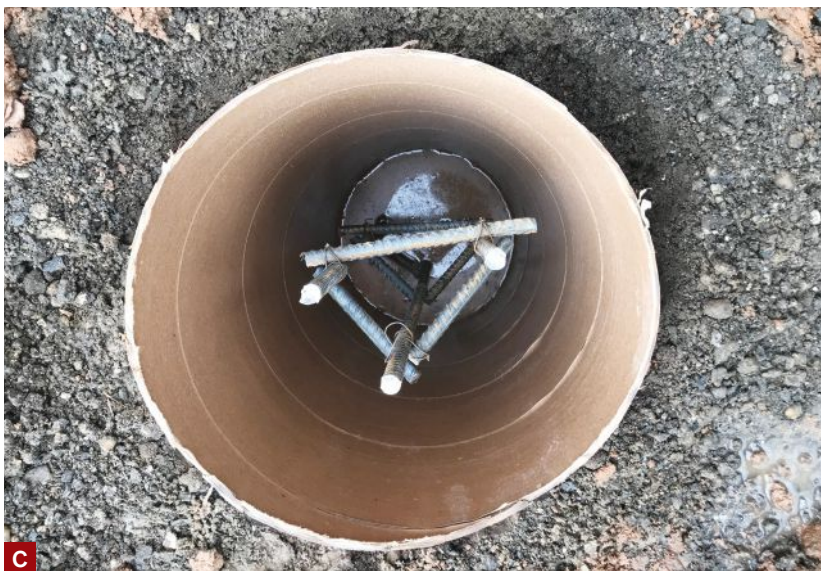
Figure 1. Workers dismantled the existing steel deck and concrete patio pads (A) and replaced an entry door (B). The six new poured-concrete deck footings were reinforced with triangular rebar cages (C).
