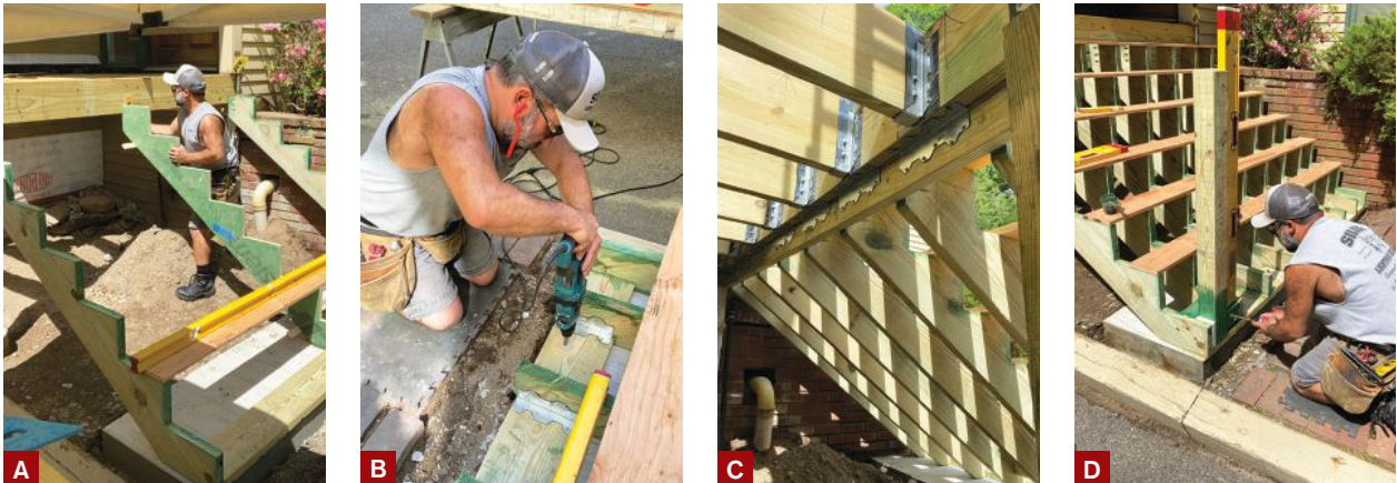
Figure 4. The author installed the end stringers first, then used the template to fine-tune the position of the remaining ones (A). The author used wedge anchors to fasten the plate to the slab (B), and metal angles to attach the dropped header for the stringers to the framing (C). Plenty of blocking was used to reinforce the landing post connection (D).
