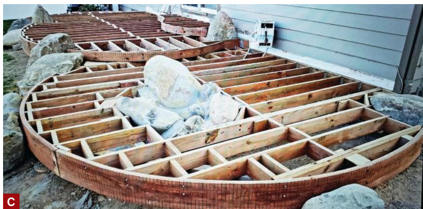
Figure 1. The existing backyard had a small concrete patio, a fire ring, and a few boulders (A). The author removed the patio and repositioned the boulders and fire ring, stabilizing them with concrete (B). The new deck frame was built over new footings and around these features, with a curved rim joist (C).
