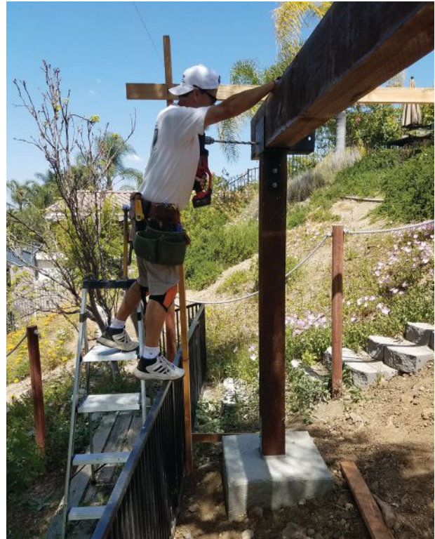
The new deck-post sizing table in the 2021 IRC offers more flexibility in deck-post design than earlier 2015 and 2018 versions of the table, as shown below.
