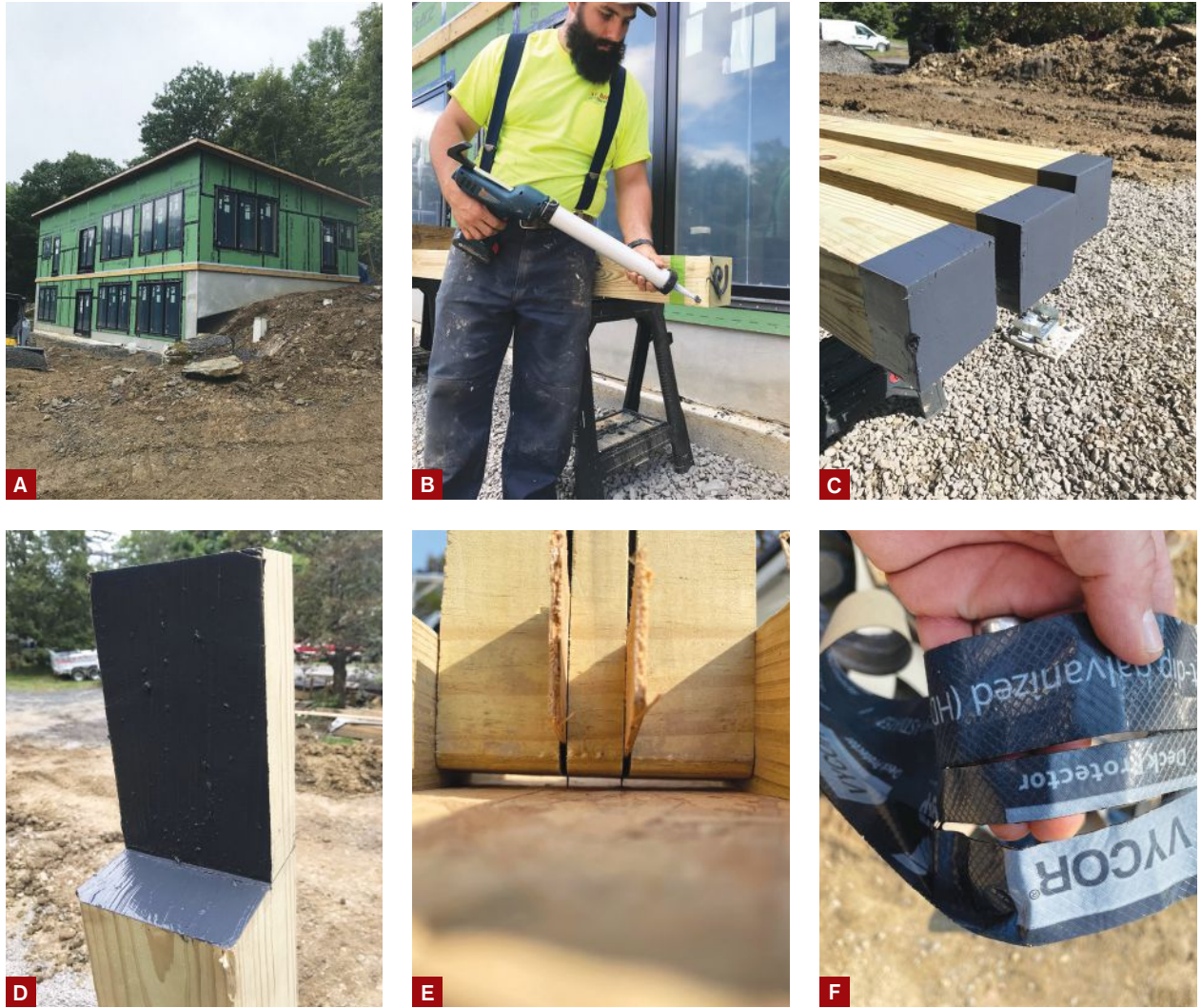
Figure 1. Precast concrete piers were installed to support the deck (A). Prior to installing the 6x6 support posts, Ed Backus applied liquid flashing membrane to the post bases (B, C) and the notches for a 2-ply dropped beam (D). Backus assembled a quick jig fitted with a couple of utility blades (E) to slice Vycor flashing tape to cover the tops of joists (F).
