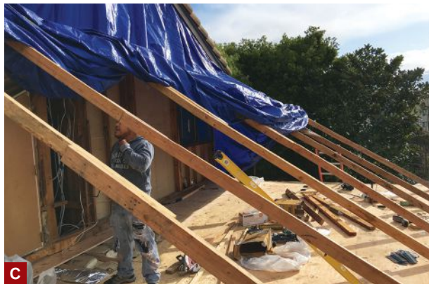
Figure 1. With most of the truss roof dismantled except for the gable end, the Pacific Ocean begins to come into view (A). Workers dismantled the roof trusses from the top down, removing the bottom chords last in order to leave the ceiling drywall intact (B). Before hanging new 9 1 / 4 -inch PSL ceiling joists, workers ripped V-shaped tapers along their top edge so that the flat-framed deck would slope toward drains installed in the center of the deck rather than toward the outside edge. While waiting for the waterproof deck membrane to be installed, workers tented the area with tarps to protect the living space below (C).
