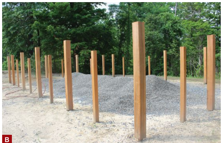
Figure 4. Alternating 6x6 and 4x4 cedar posts were installed in the garden area; here, they have been aligned, plumbed, and braced, and are ready for concrete (A). In this area, the fence design required taller, 6x6 cedar posts with three stainless steel cables run between them at the top to prevent deer from bounding into the garden (B).
