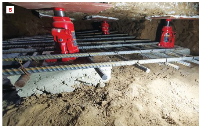
Moment frame. One of the two concrete pillars supporting a Z-shaped lintel (2). Column layout for the new moment frame, south corner (3). A crew member begins work accessing the existing north footing (4). “Sacrificial” bottle jacks are used to support the existing footing during footing underpinning (5).
