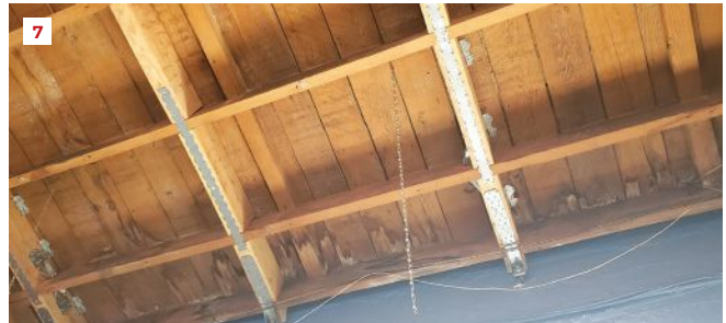
Roof connections. Crew members sister new 2x8s onto existing rafters at steel angle diagonal brace locations above the storefront entry (6). Between rafters parallel to the wall, 4-by blocking was added and secured with metal strapping and tension ties (7).
