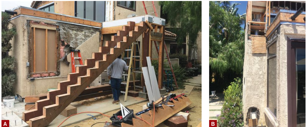
Figure 3. To seismically reinforce the stairs, workers connected a grade beam at the lower landing to the moment-framed upper landing with stringers cut from 4x14 treated Douglas fir beams (A). The chimney was reconfigured to make room for a new direct-vent gas fireplace for the rooftop deck and reframed as a low privacy wall (B).
