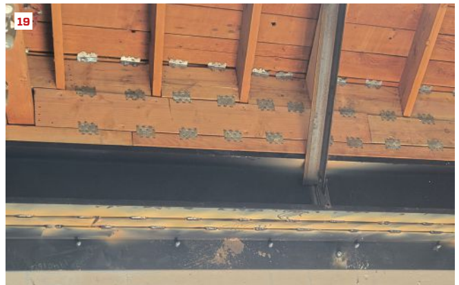
Roof connections. Completed structural work at the angled, wall-to-wall storefront opening includes the steel angle lintel, steel angle diagonal bracing, 2-by blocking, and metal connectors (18, 19).
