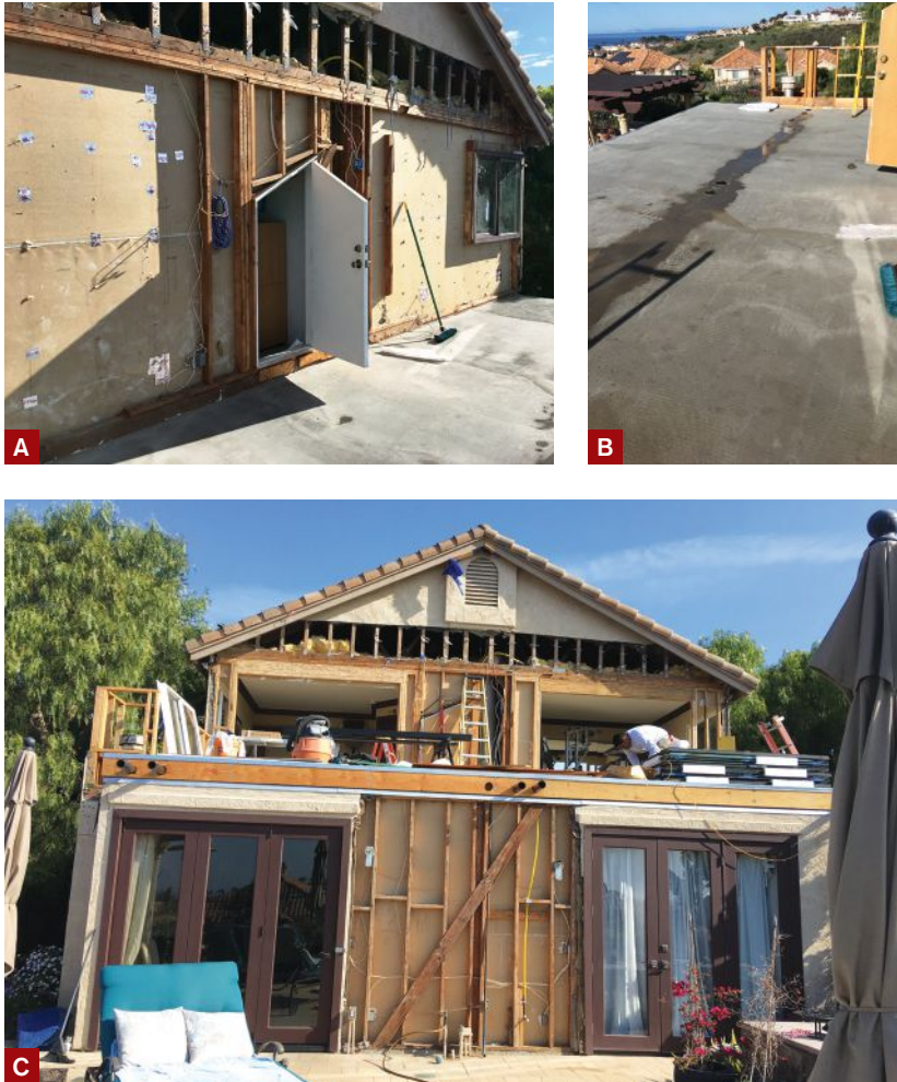
Figure 2. The roof deck was finished with a three-coat stucco finish over diamond lath stapled to the sheathing, followed by a Silcor liquid-applied waterproofing membrane system (A). Water drains through three pairs of roof drains oriented along the centerline of the deck (B). Once the new deck was watertight, workers reframed the wall to install two new bi-fold doors to match the doors on the first floor (C).
