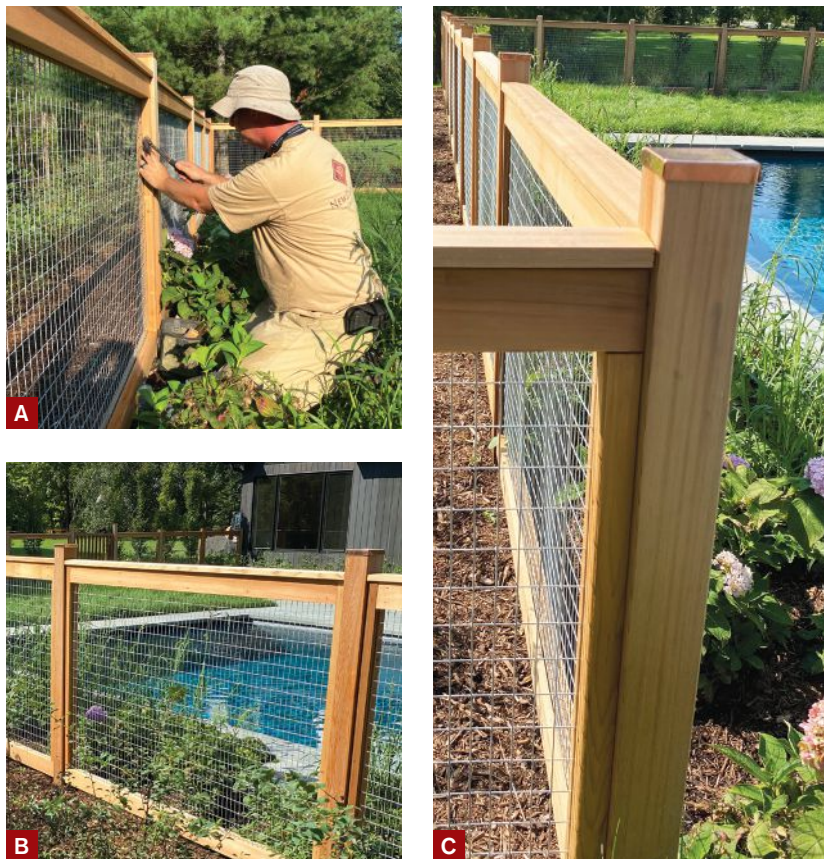
Figure 5. Workers prefabricated cedar fencing panels, sandwiching galvanized welded wired mesh between a 2x4 frame and a 1-by face frame, and then fastened them to the posts with stainless steel screws (A, B). The posts were topped with site-fabricated copper caps (C).
