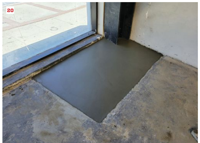
Moment frame. A second concrete pour buries the column base plates and is troweled smooth (20).
