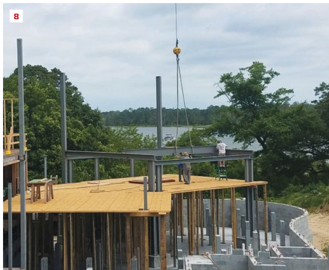
The framing crew erected an extensive temporary scaffolding system over a future outdoor living pavilion to install the complex steel framing for the master suite (B).
