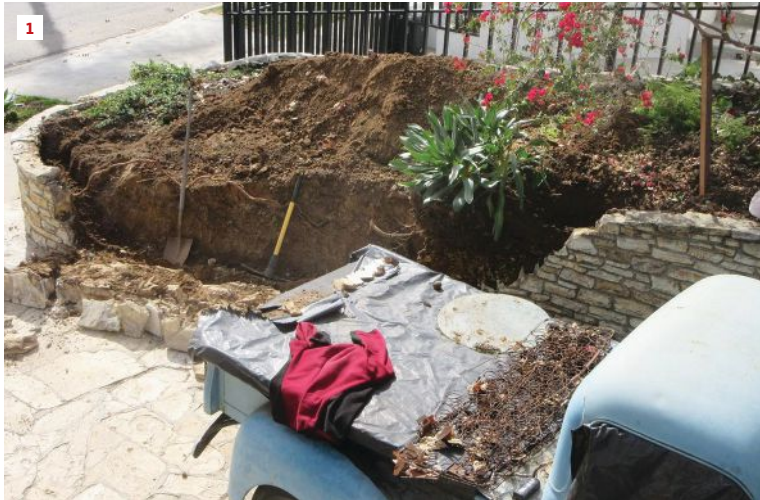
The middle third of a leaning, unreinforced stone retaining wall collapsed during excavation by the homeowner (1).
