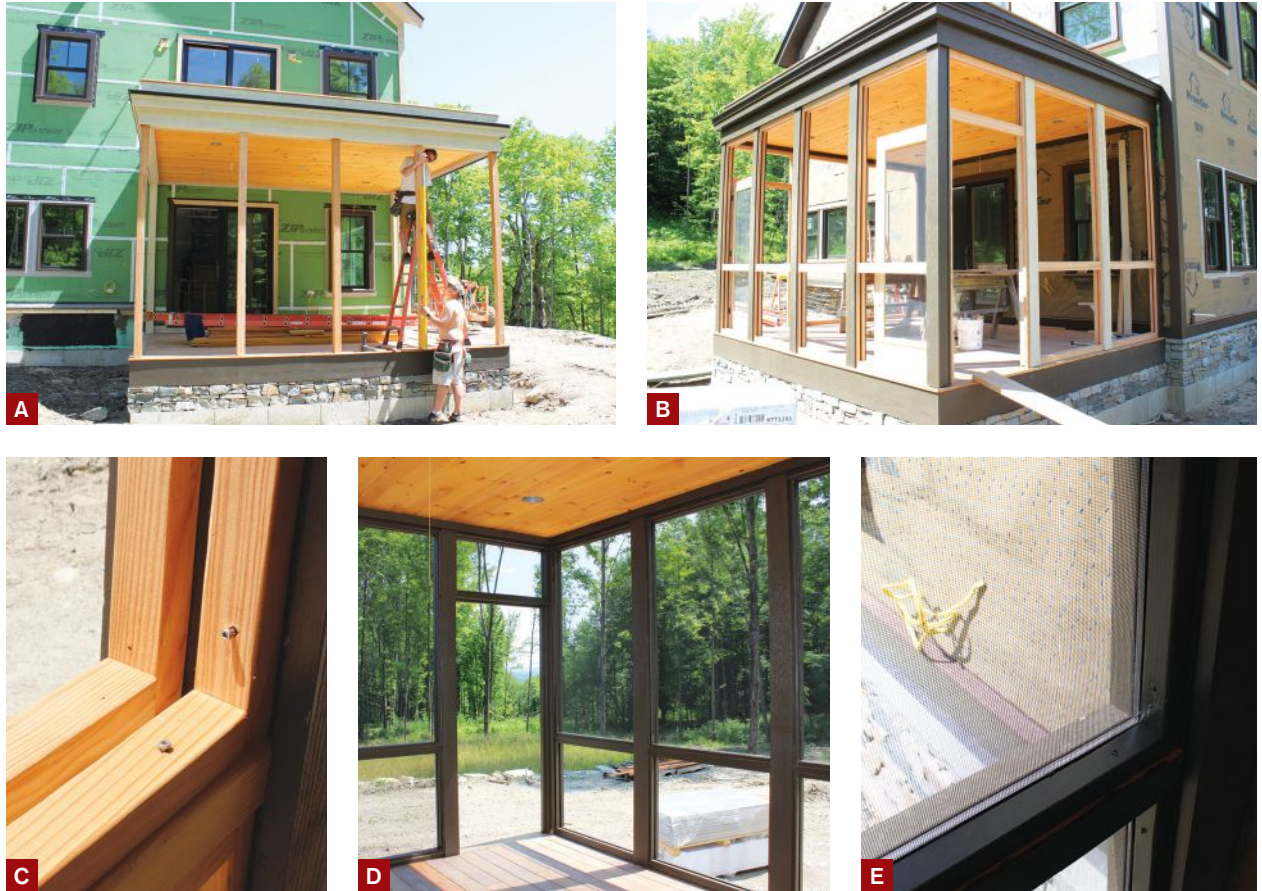
Figure 4. Additional 4x4 posts were installed to frame the openings for the screen panels and doors (A). Prior to screen installation, the trim was painted to match the trim on the rest of the house (B). Fixed (on the exterior) and removable (on the interior) red-cedar stops were added to the openings (C) in preparation for the aluminum screen panels (D, E).
