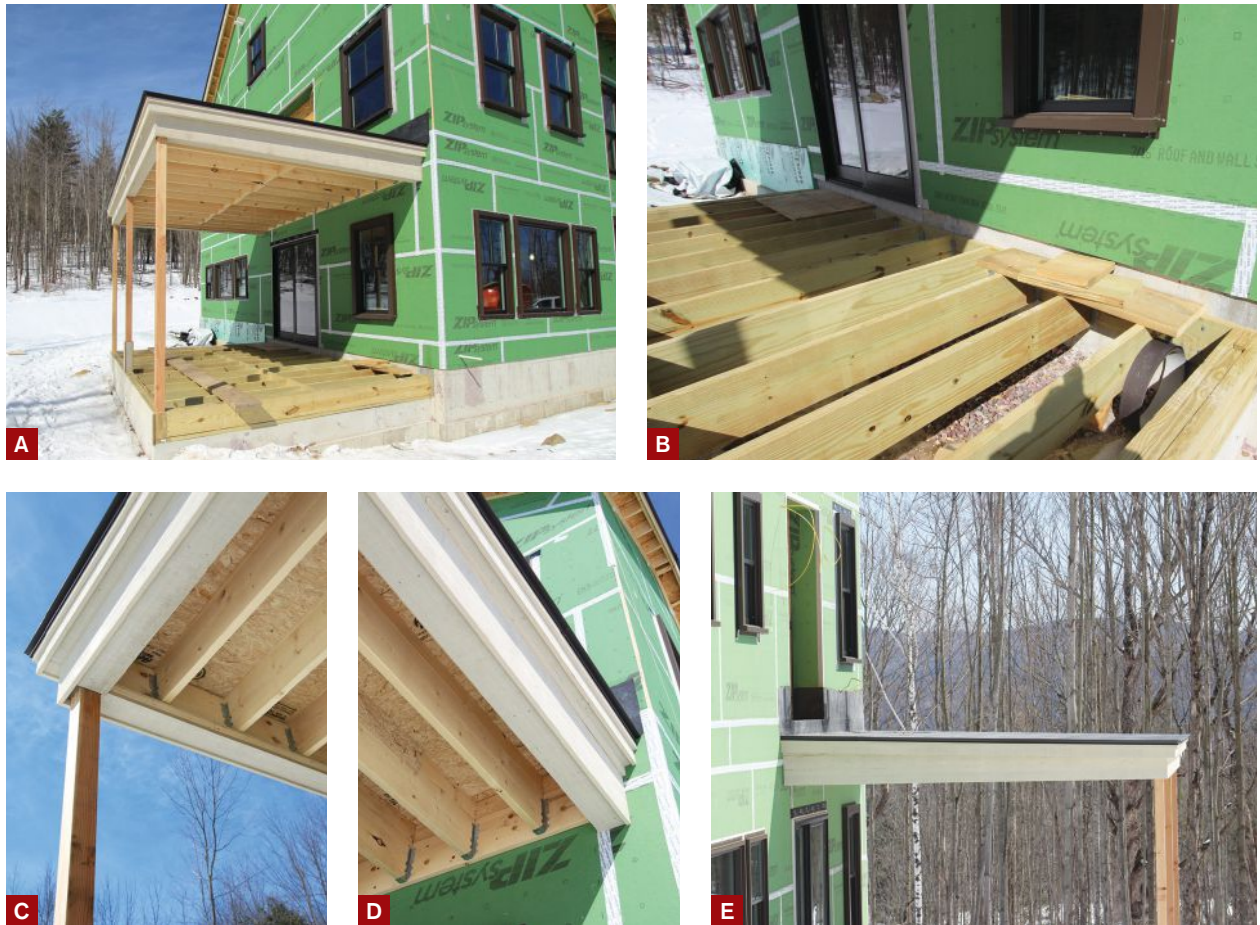
Figure 1. The screened porch was conventionally framed like a deck with pressure-treated lumber but supported by a poured concrete stem-wall foundation rather than posts or piers (A). The deck ledger was bolted to the home's concrete foundation with wedge anchors (B). Tapered rippings added to the ceiling joists (C, D) created the pitched roof deck (E).
