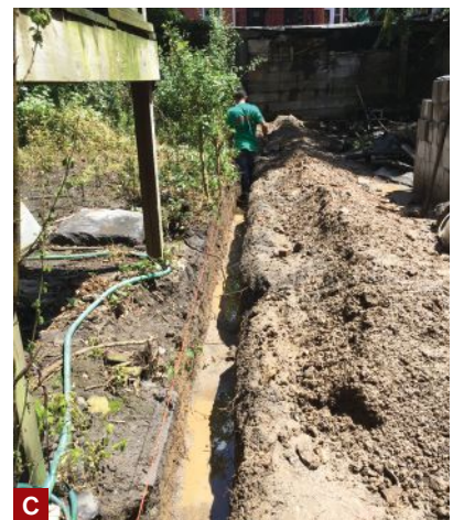
Figure 1. Measuring just 15 feet wide, the overgrown backyard was bordered on two sides by an old cyclone fence (A). After removing it, workers removed the sod and brought in materials to build a short CMU retaining wall around the yard and a perimeter fence (B). With no access for machinery, the trench for the perimeter fence was dug by hand (C).
