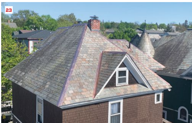
Salvaged semi-weathering green-gray slate blends into the existing slate on a finished open valley (21), dormer (22), and north- and west-facing sections of roof (23). Seventy-five percent of the existing slates were left intact.
