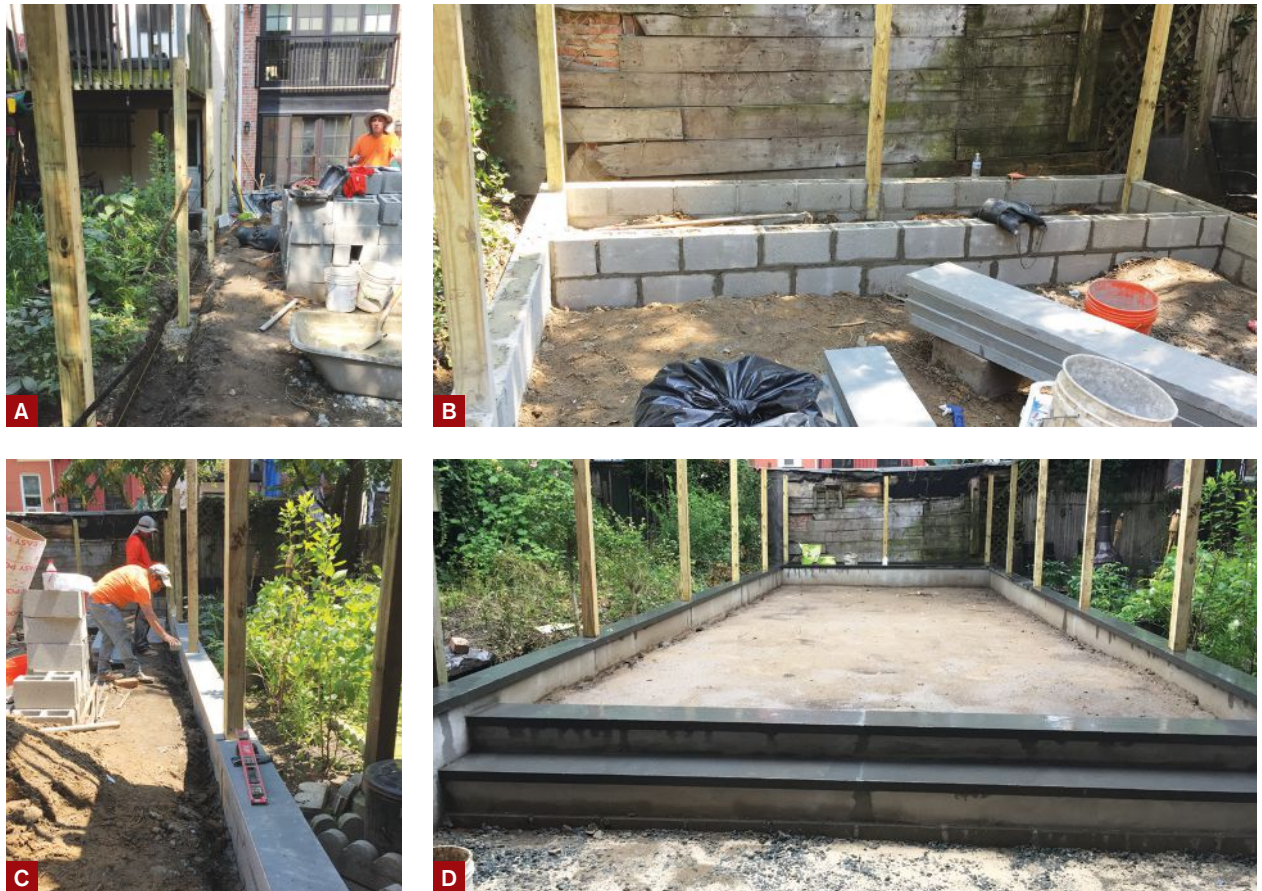
Figure 2. The 4x4 posts for the perimeter fence were set in 3-foot-deep holes that were then filled with concrete (A). Over a compacted gravel base in the bottom of the trench, masons laid up a short CMU wall around the perimeter of the yard, as well as a wall to create a small planting bed at the back of the yard (B). The walls were capped with bluestone (C). Bluestone treads were installed on the steps leading down to the lower level near the house (D).
